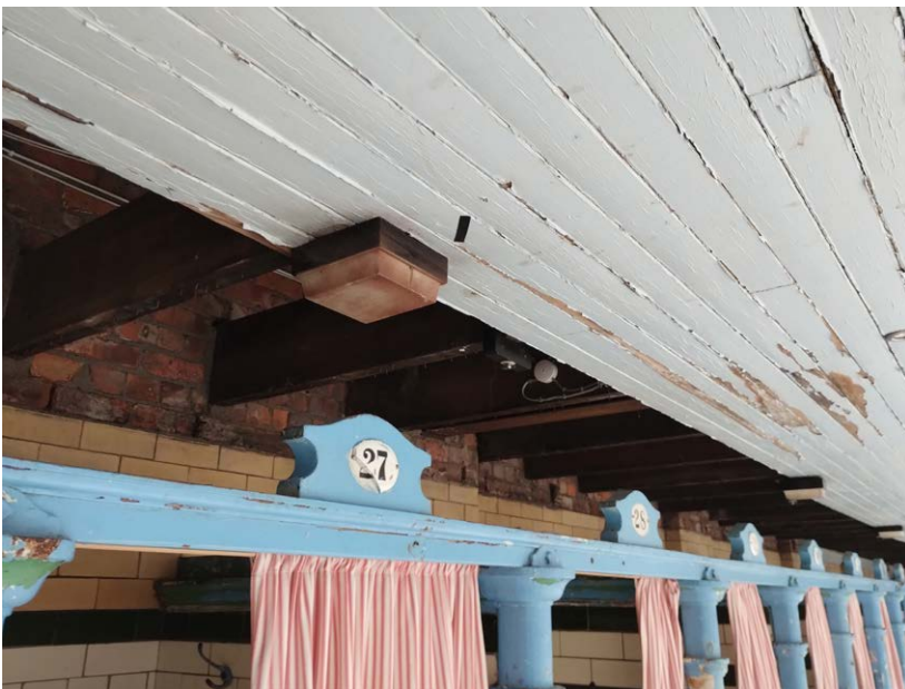
Existing Emergency Lighting
