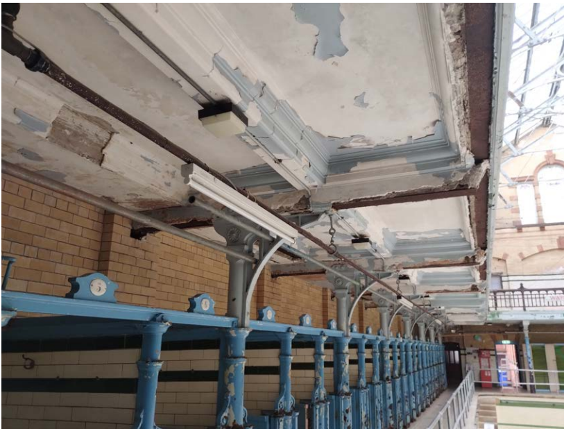
Existing Emergency Lighting
