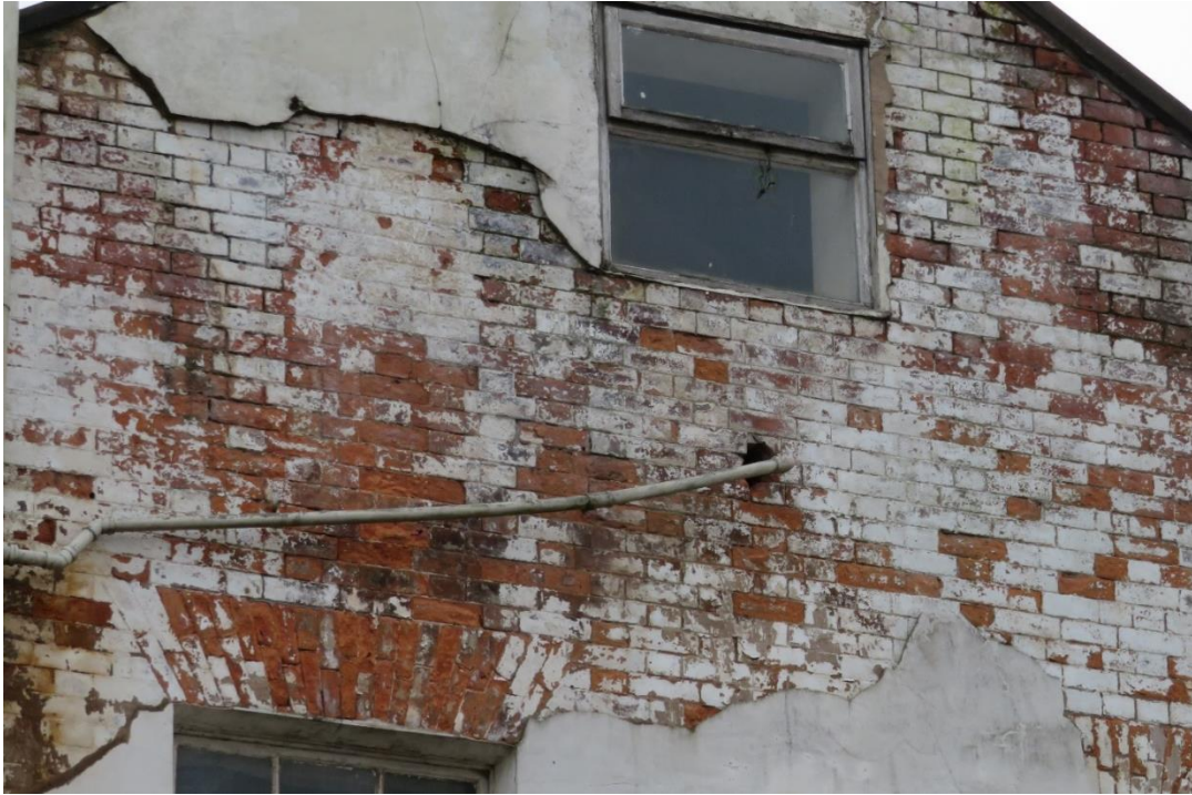
Close-up of damaged faces to the voussoirs and bricks above the first floor window and at eaves level.
