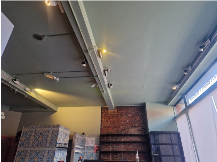
CEILING AND LIGHTING
