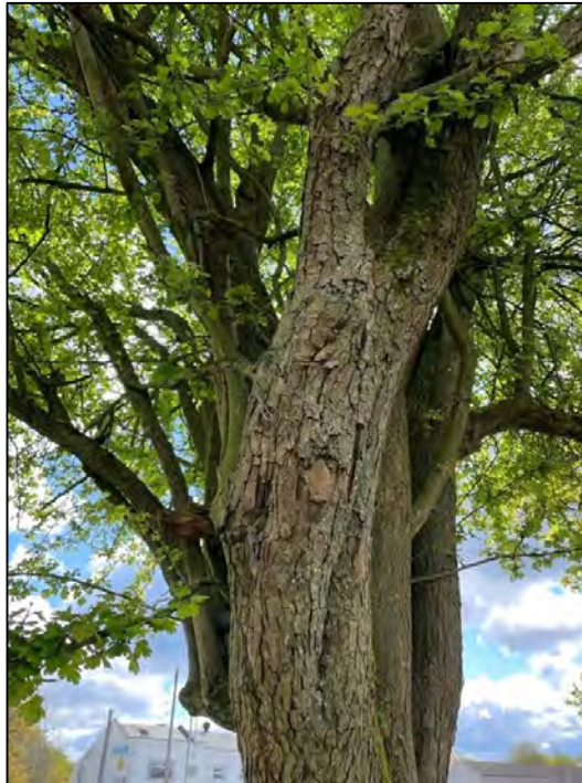
Plate 16: Loose and lifted bark on T4
