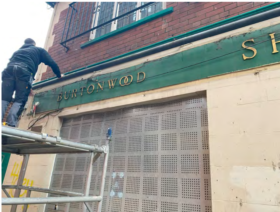
Plate 12 – Faience fascia exposed following removal of modern fascia signage board.
