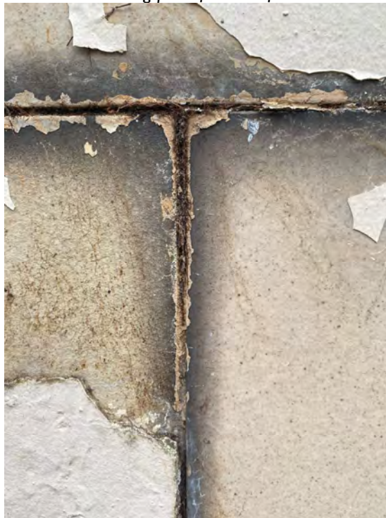
Plate 8 – Original faience finish with typical defects to the arrises of the block.
