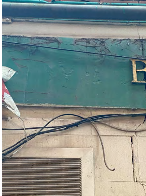
Plate 13 – ‘Scars’ of hacked offer relief lettering to the faience fascia to Silk Street.
