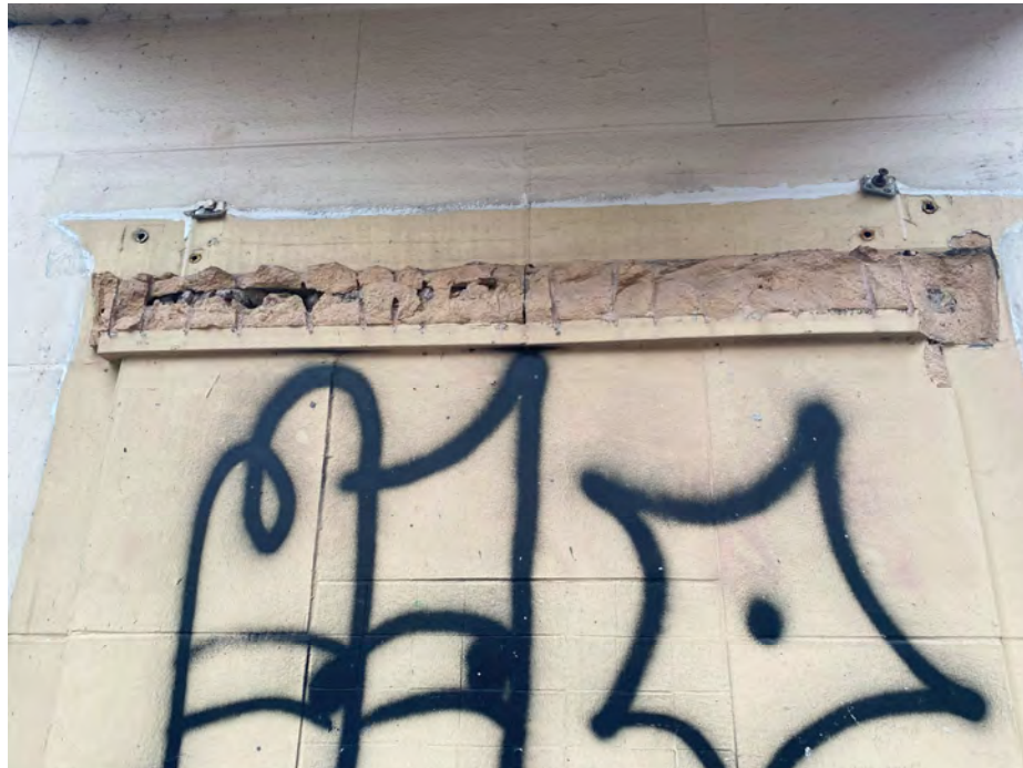
Plate 10 – Damage to faience sign to the splayed northwest corner.
