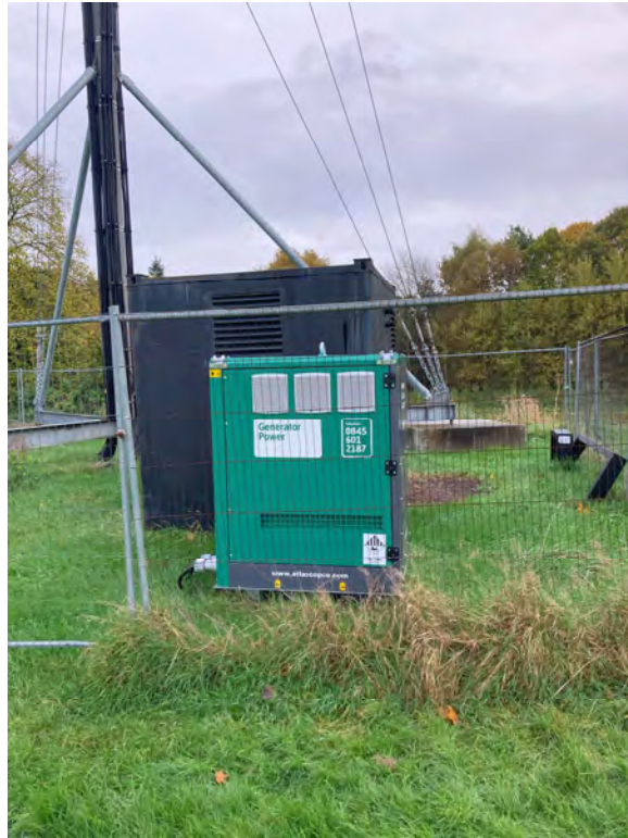
Photo 3: Power Generator Located on Site
