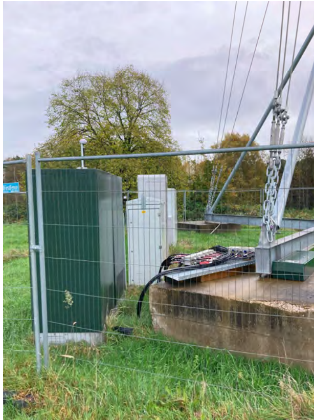
Photo 5: Electrical Wiring on Site
