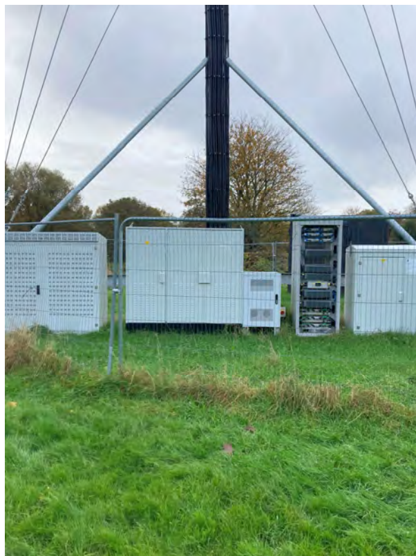
Photo 4: Electrical Equipment Surrounding Telecoms Mast
