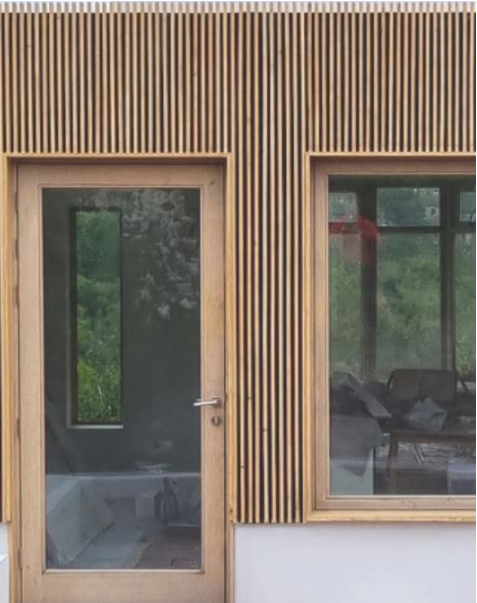
Timber windows and doors
