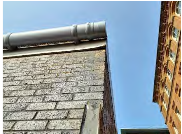
Photograph 10: External potential roost feature (PRF) on north-west aspect along Newton Street between the wooden fascia and brick wall.
