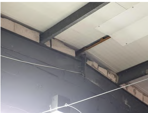
Photograph 7: Gaps between internal dividing wall and ceiling.
