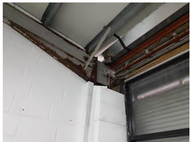
Photograph 8: Gap between internal dividing wall and ceiling.
