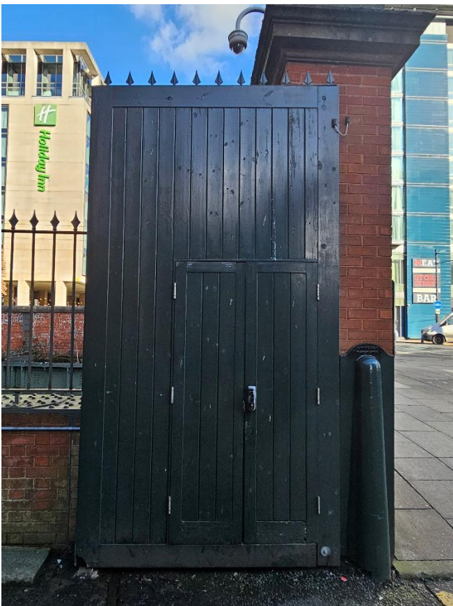
Existing gates in open position, with areas of decay clearly visible
