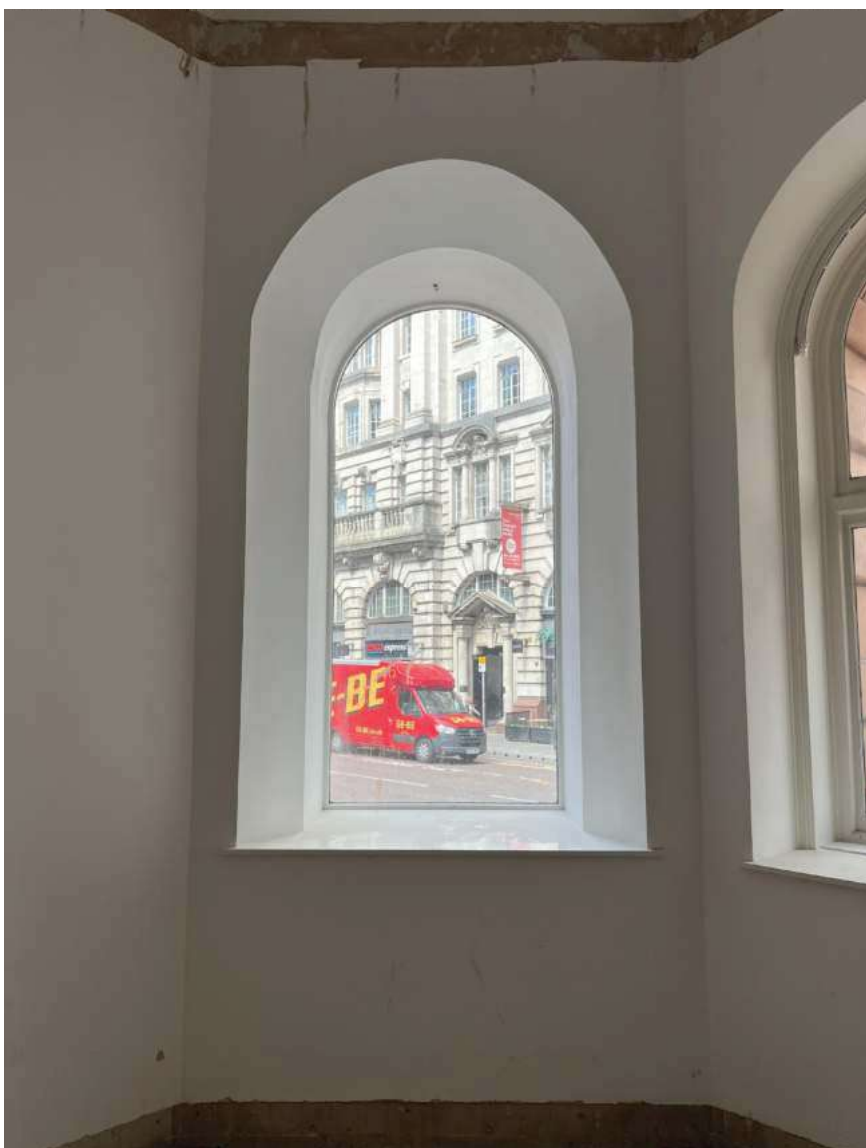
11 EXISTING PHOTOGRAPH 141 NTS EX CORNER WINDOW TO BE REPLACED
