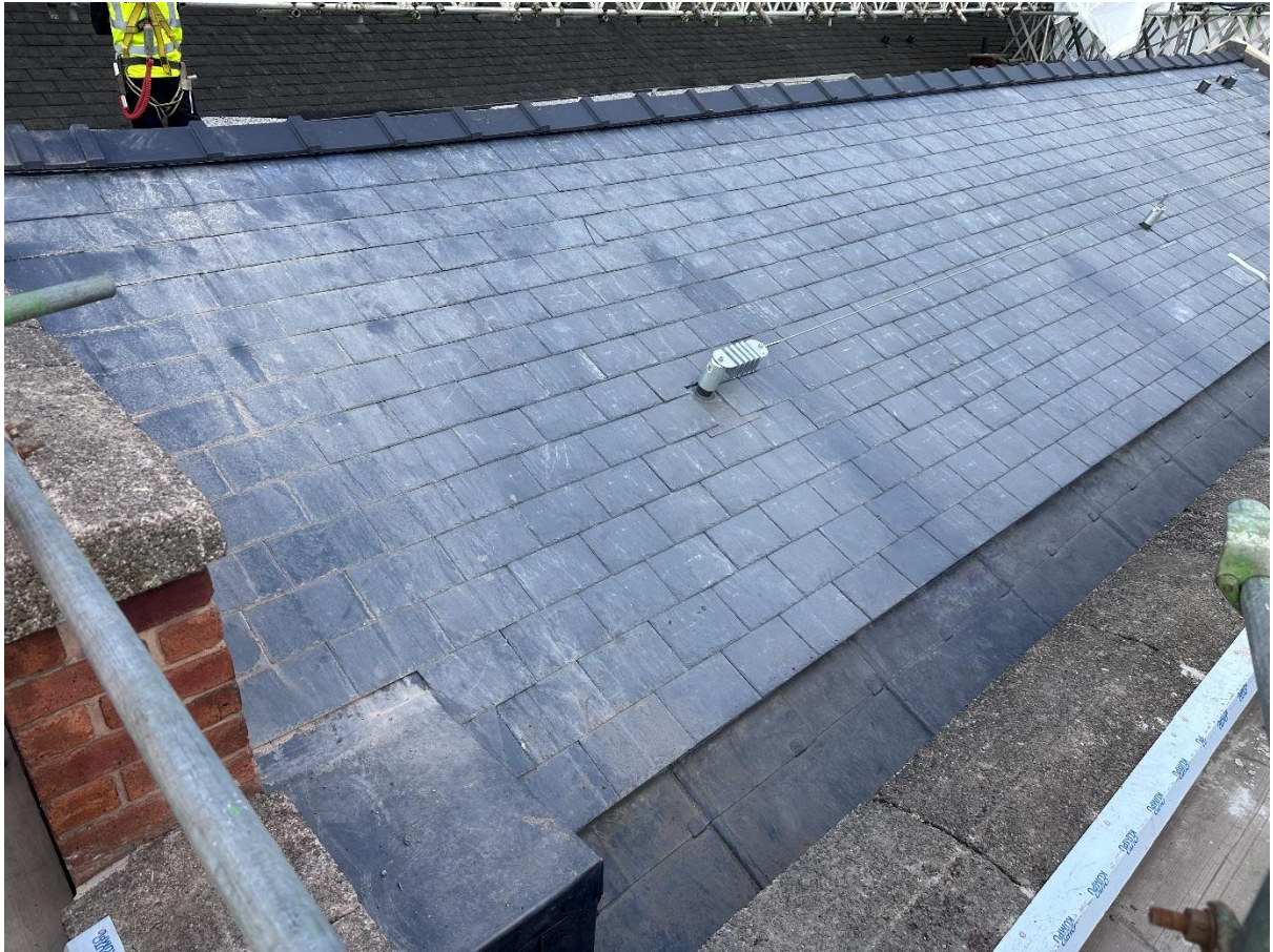
Installed guided fall arrest system
