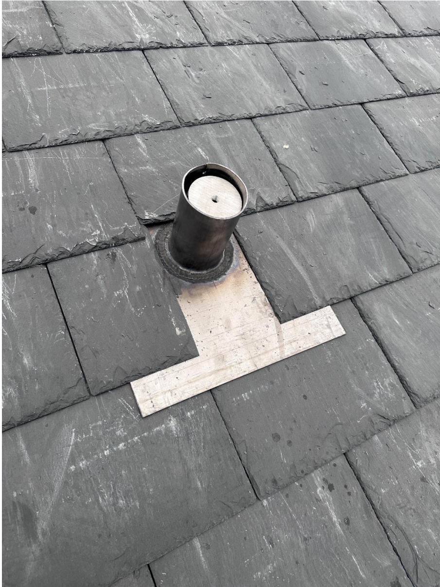
Independent gantry / walkway fixing points with lead flashing and shroud
