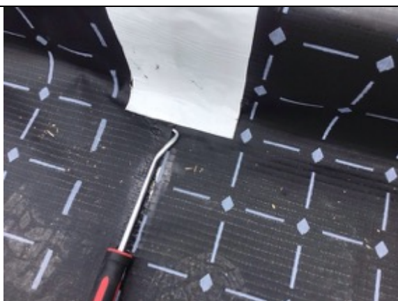
Recorded weld defect on plot 1
