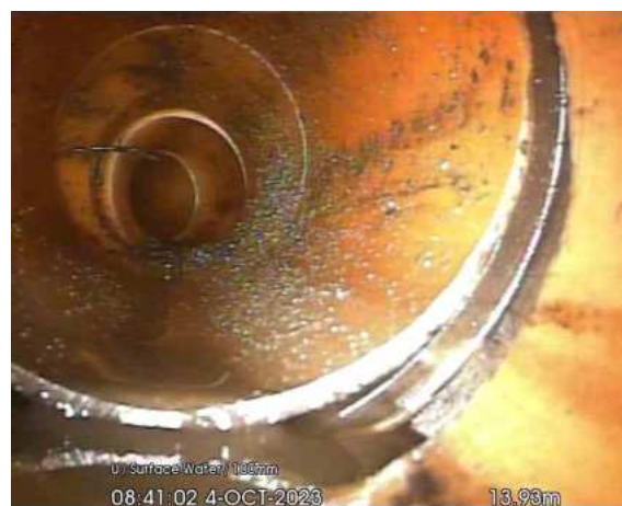
MH3 US ACO_13-93m_084102.jpg, 00:01:23, 13.93 m Joint displaced, large
