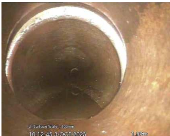
MH19 US GULLY_1-89m_101245.jpg, 00:00:16, 1.89 m Joint displaced, medium
