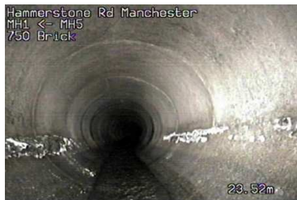
MH1X_012cdac9-bc28-4f1c-bf1c-46af3d245a1e_20240201_1 01857_282.jpg, 00:03:13, 23.52 m Attached deposits, grease at 08 o'clock, 5% cross-sectional area loss, grease
