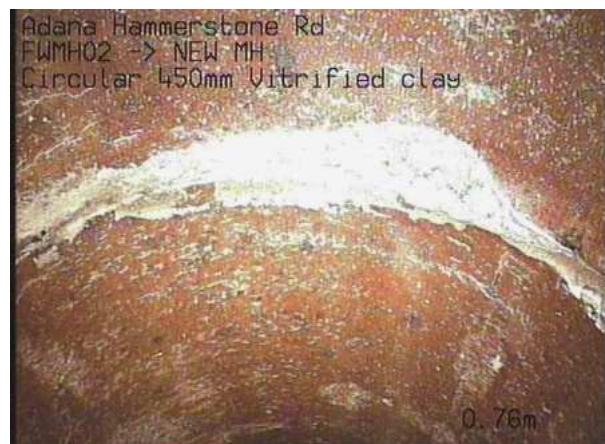
FWMH02X_d2215c8f-f3bb-4127-9b8e-fde0659868d8_20230929_124600_242.jpg, 00:01:26, 0.76 m Attached deposits, encrustation from 7 o'clock to 5 o'clock, 5% cross-sectional area loss, start
