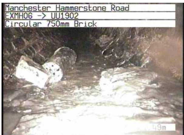
EXMH06X_705dcd75-53f9-4874-8eb6-03ca64d7bcdd_20230704_092405_783.jpg, 00:02:25, 21.52 m Attached deposits, encrustation from 5 o'clock to 7 o'clock, 15% cross-sectional area loss, Bricks are catching on this whilst jetting, unable to remove
