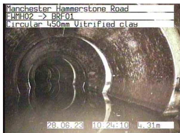
FWMH02X_a9c62bf7-3e55-45f3-a47c-e56f0c333b3e_20230704_091900_013.jpg, 00:02:25, 4.31 m Line deviates left, start
