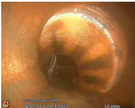
MH4 DS MH5_16-69m_141551.jpg, 00:01:10, 16.69 m Joint displaced, medium
