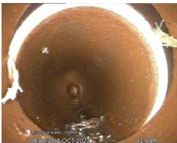
MH3 US ACO_12-04m_084036.jpg, 00:01:08, 12.04 m Joint displaced, large
