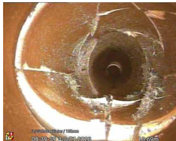
MH3 US ACO_10-69m_083959.jpg, 00:00:48, 10.69 m Fractures, multiple at 12 o'clock
