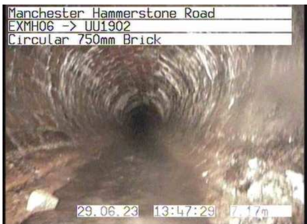
EXMH06X_eed5b47b-ed46-48a0-857e-6e44c42f80e7_20230704_092341_194.jpg, 00:00:36, 7.27 m Settled deposits, coarse, 5% cross-sectional area loss
