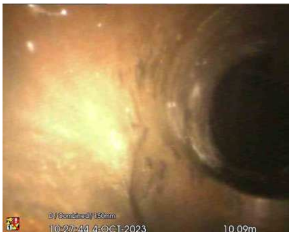
MH25 DS UU2801_10-09m_102744.jpg, 00:01:27, 10.09 m Junction at 6 o'clock, 150mm dia, DROP SHAFT
