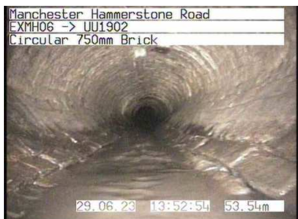
EXMH06X_b2d37cc8-baa6-4236-ae01-568821f6fe03_20230704_092421_558.jpg, 00:06:00, 53.59 m Attached deposits, encrustation from 8 o'clock to 4 o'clock, 5% cross-sectional area loss, start
