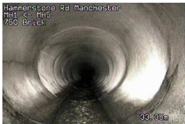
MH1X_51f353b9-360a-4272-9ee9-2f0bf5299c1e_20240201_1 02217_287.jpg, 00:04:10, 14.00 m Fracture, longitudinal at joint at 9 o'clock
