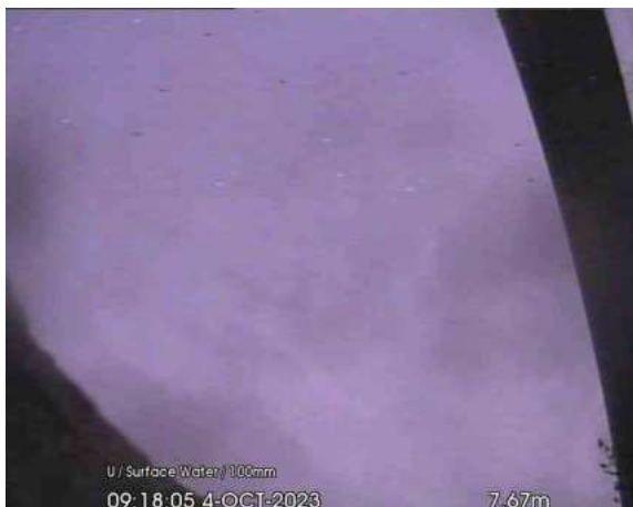
MH16 US ROD EYE_7-67m_091805.jpg, 00:00:34, 7.67 m Finish node, rodding eye, reference: ROD EYE, NO CAP ON RE
