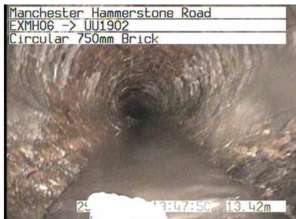
EXMH06X_a55d7d83-2f42-41d3-88d7-abd184265b1f_20230704_092346_033.jpg, 00:00:56, 13.44 m Settled deposits, coarse, 5% cross-sectional area loss
