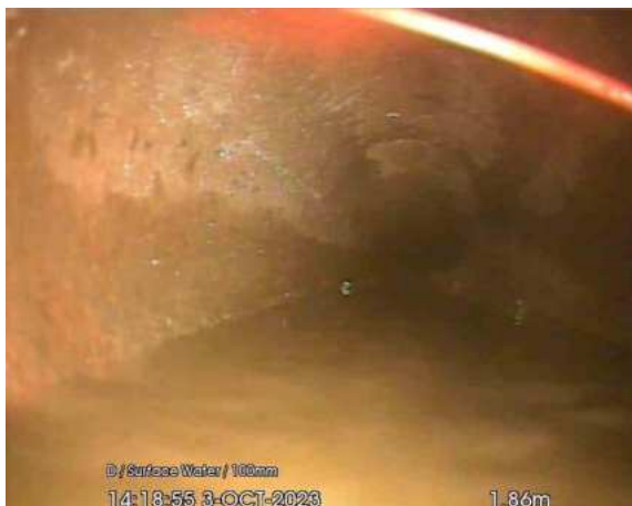
MH4A DS MH5_1-88m_141855.jpg, 00:00:11, 1.88 m Other obstacles at joint from 10 o'clock to 3 o'clock, 5% cross-sectional area loss, PLASTIC
