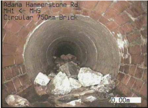
MH1X_1e4fff8e-f462-4aec-b3d1-adf4e246590f_20230928_14 4150_540.jpg, 00:01:02, 0.00 m Settled deposits, hard or compacted, 40% cross-sectional area loss, Rocks & Bricks ahead
