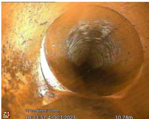
MH24 DS_10-78m_101357.jpg, 00:00:41, 10.78 m Joint displaced, medium
