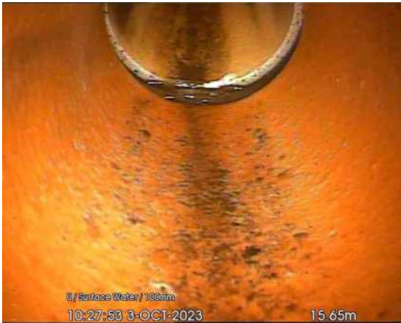
MH28 US RWP B_15-65m_102753.jpg, 00:01:41, 15.65 m Survey abandoned, RWP B
