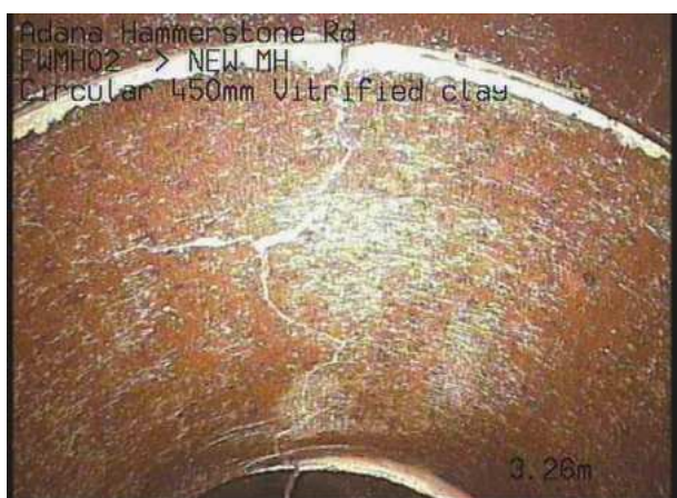
FWMH02X_d67fa18a-261f-42cc-b472-823572ada9df_20230929_124648_735.jpg, 00:02:12, 3.26 m Fracture, longitudinal at 12 o'clock, start
