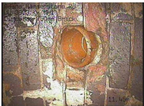
UU 3803X_2d64c7c1-4914-4176-8e85-39894b60b95c_20230929_110716_314.jpg, 00:01:37, 11.45 m Connection other than junction at 1 o'clock, 150mm dia
