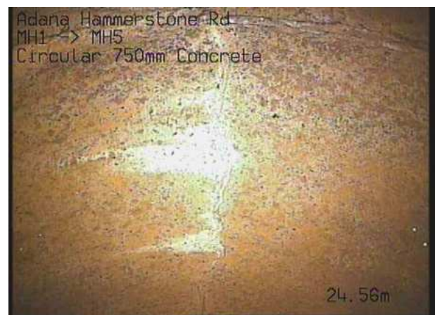
MH1X_3d9dbc05-6e24-48b4-bd28-cb39d0947a73_20230929_082952_988.jpg, 00:06:57, 24.56 m Fracture, longitudinal at 12 o'clock, start
