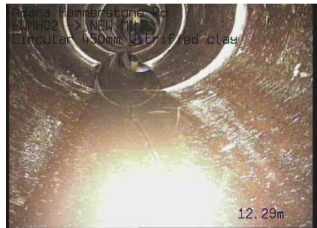
FWMH02X_f3b58675-fd07-4717-8b15-d7f2aa510cb6_20230929_125036_729.jpg, 00:06:02, 12.29 m Fracture, longitudinal at 6 o'clock
