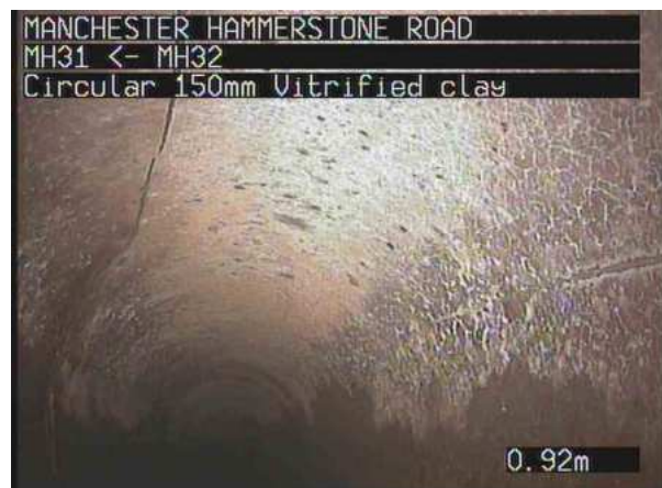
MH31X_a7e1bd3b-4274-4a7a-8eac-753dbce24893_20230822_142250_429.jpg, 00:00:24, 0.90 m Fracture, longitudinal at joint at 11 o'clock
