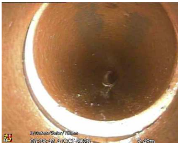
MH3 US ACO_9-49m_083943.jpg, 00:00:41, 9.49 m Joint displaced, medium
