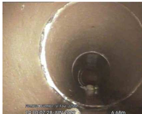
FWMH01X_fca69c75-ec5f-4891-b983-80ffa3de1089_20230704_091625_459.jpg, 00:00:43, 6.68 m Settled deposits, coarse, 5% cross-sectional area loss
