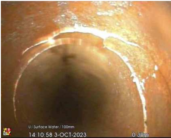
MH4 US GULLY_0-30m_141058.jpg, 00:00:04, 0.30 m Fractures, multiple at joint from 8 o'clock to 5 o'clock
