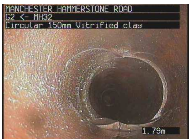
G2X_747da227-0512-4bbe-84f2-efa2331e3276_20230822_14 4655_798.jpg, 00:01:08, 2.30 m Deformed sewer or drain, 10%
