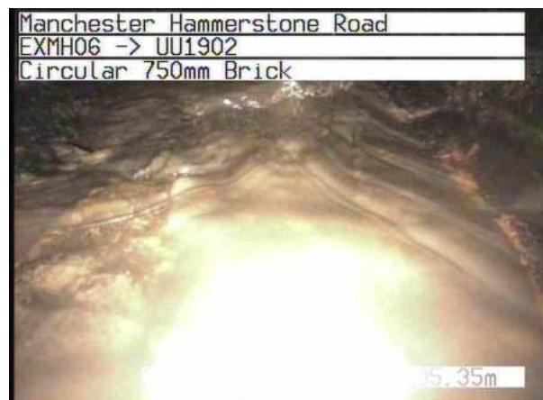
EXMH06X_db1f7b05-343a-4923-9bc0-7baf1208481a_20230704_092412_620.jpg, 00:04:43, 35.12 m Deformed horizontally, 5%, Bricks moved causing an improper flow
