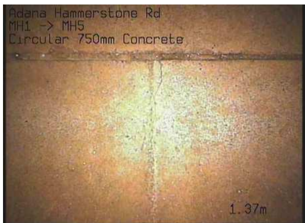
MH1X_e8ddb24d-3b20-4023-afa7-0dde4b1c943f_20230929_082331_720.jpg, 00:00:36, 1.37 m Fracture, longitudinal at 12 o'clock, start
