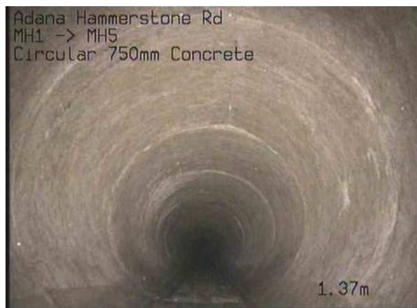
MH1X_3c9c27db-fb99-4094-9bf2-97fcb271940e_20230929_082340_048.jpg, 00:00:36, 1.37 m Fracture, longitudinal at 12 o'clock, start
