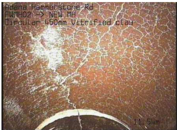
FWMH02X_633f7784-7216-4371-80bf-317db178d39e_20230929_125002_555.jpg, 00:05:27, 11.54 m Fracture, longitudinal at 12 o'clock, start
