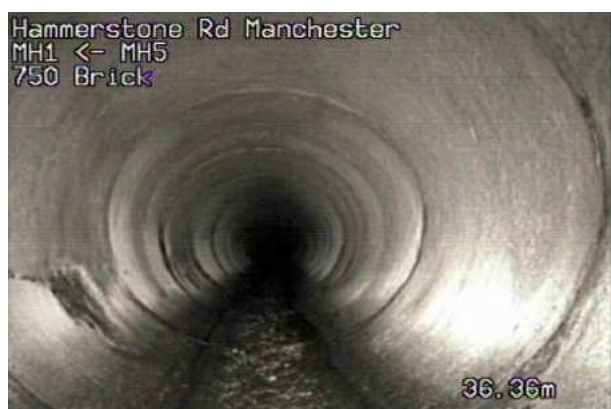
MH1X_d86746ce-af0b-49ac-bf60-ade12876c7f0_20240201_1 02241_993.jpg, 00:04:23, 37.00 m Fracture, longitudinal at joint at 8 o'clock
