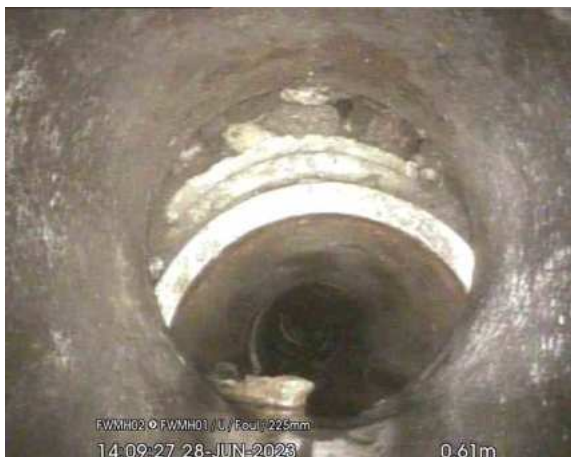
FWMH02 US FWMH01_0-61m_140927.jpg, 00:00:15, 0.61 m Joint displaced, large
