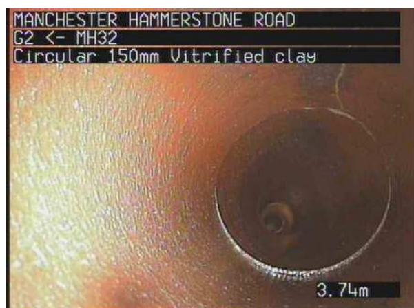
G2X_ab06da00-461d-487a-9062-864238af2135_20230822_1 44730_122.jpg, 00:01:49, 3.74 m Fracture, longitudinal at joint at 1 o'clock
