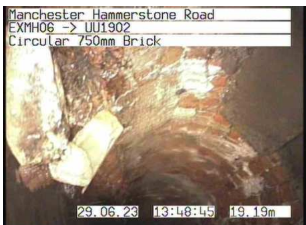
EXMH06X_1122bd28-ce2d-4a72-aa66-86907662bf99_20230704_092352_690.jpg, 00:01:51, 19.18 m Other obstacles, brick or masonry in invert from 7 o'clock to 8 o'clock, 15% cross-sectional area loss, Unable to jet due to bricks catching encrustation
