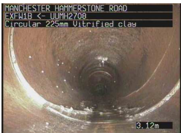
EXFW1BX_4dbb72b1-1295-4541-a76e-22125fdc992b_20230822_110208_059.jpg, 00:00:46, 3.09 m Fracture, circumferential at joint from 1 o'clock to 10 o'clock
