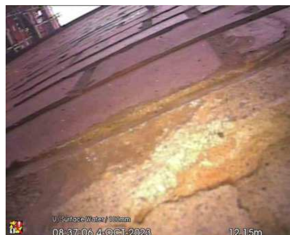
MH3 US RWP_12-15m_083706.jpg, 00:01:02, 12.15 m Survey abandoned, RWP MISSING OFF WALL
