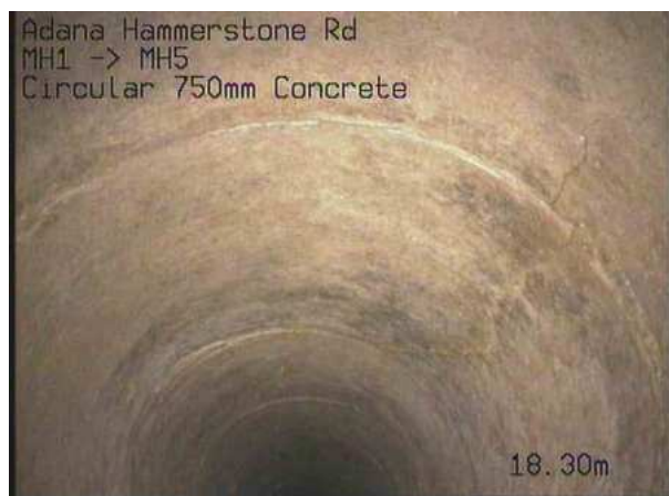
MH1X_c2594daa-fcaf-402d-bd67-0043181de174_20230929_082633_141.jpg, 00:03:37, 18.30 m Fracture, longitudinal at 2 o'clock, start
