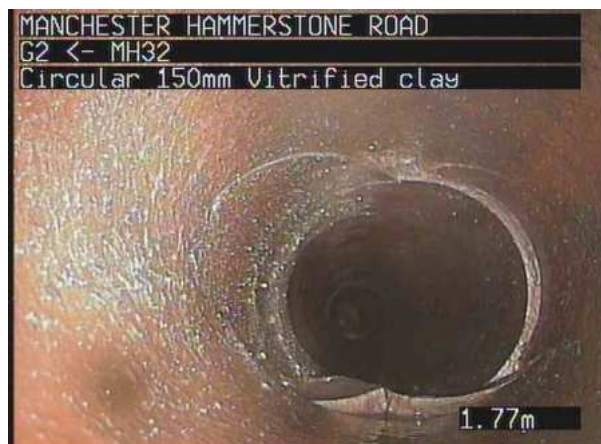
G2X_2be08d98-3f9c-4bdc-8a9a-d6455144f56f_20230822_14 4653_113.jpg, 00:01:03, 2.30 m Broken pipe from 4 o'clock to 8 o'clock
