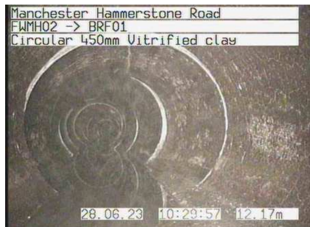
FWMH02X_a5d1eb1f-37c1-4bc2-8a2e-f654ab212450_20230 628_103631_547.jpg, 00:08:01, 12.17 m Fracture, longitudinal at joint at 12 o'clock
