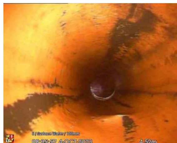
MH3 US RWP_4-52m_083557.jpg, 00:00:25, 4.52 m Deformed sewer or drain, 10%
