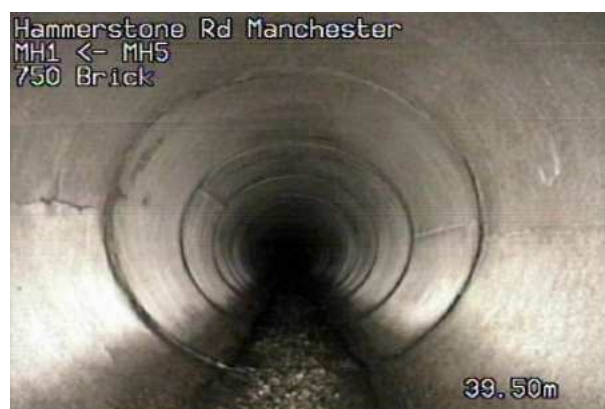
MH1X_cd383f44-f452-42c0-b12e-c7d4cdfae8e6_20240201_1 02311_947.jpg, 00:04:38, 40.00 m Fracture, longitudinal at joint at 9 o'clock
