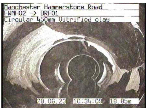
FWMH02X_7d793936-b1e4-4fb6-b0b0-916719dee72a_20230 704_092158_557.jpg, 00:12:19, 18.85 m Broken pipe from 8 o'clock to 4 o'clock
