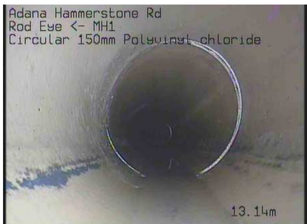
Rod EyeX_89df72d6-3b80-41c3-8f57-19804605fbd5_20231002_1 10348_578.jpg, 00:01:22, 13.14 m Deformed sewer or drain, 30%
