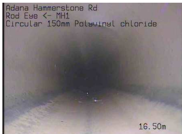
Rod EyeX_ccd54a6e-8f3a-4a5b-afef-6d8136f2e6f5_20231002_110 406_458.jpg, 00:01:41, 16.50 m Deformed sewer or drain, 5%
