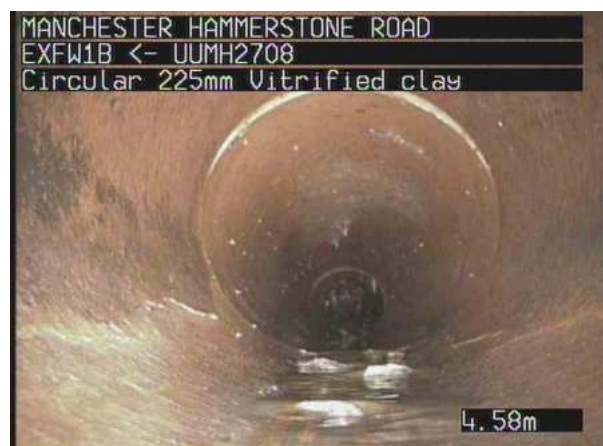
EXFW1BX_db974e72-2cce-4a01-80a6-9243de8bc956_20230822_110300_543.jpg, 00:01:32, 4.58 m Fracture, longitudinal at 4 o'clock
