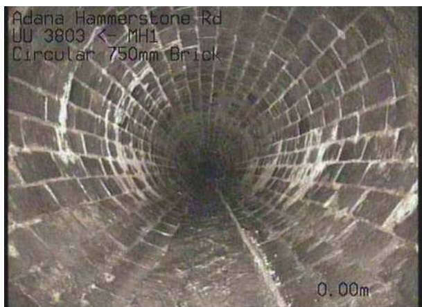
UU 3803X_7c4fe95a-6172-400c-8e55-e9b46b12f59b_20230929_110556_997.jpg, 00:00:17, 0.00 m General remark, rope running along invert
