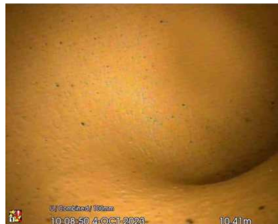
MH24 US_10-41m_100850.jpg, 00:01:26, 10.41 m Survey abandoned, UNABLE TO PASS BENDS
