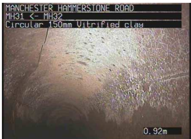
MH31X_56cae0d2-2bc6-4c28-862c-216765a5cfea_20230822_142250_192.jpg, 00:00:24, 0.90 m Fracture, longitudinal at joint at 11 o'clock
