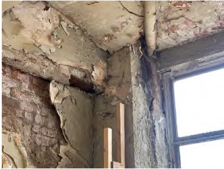
Figure 6: Water Ingress - Fourth Floor
