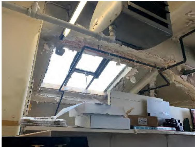
Figure 5: Water Ingress - Fourth Floor
