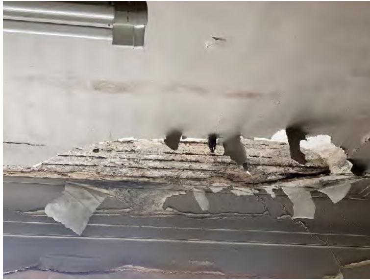
Figure 14: Exposed Reinforcement - Seventh Floor
