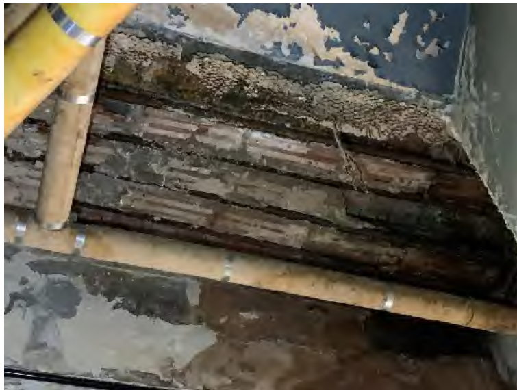
Figure 13: Exposed Reinforcement - Sixth Floor
