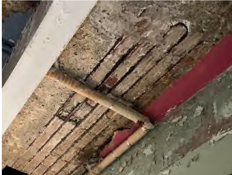
Figure 12: Exposed Reinforcement - Sixth Floor
