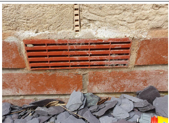
4. Air brick on site.
