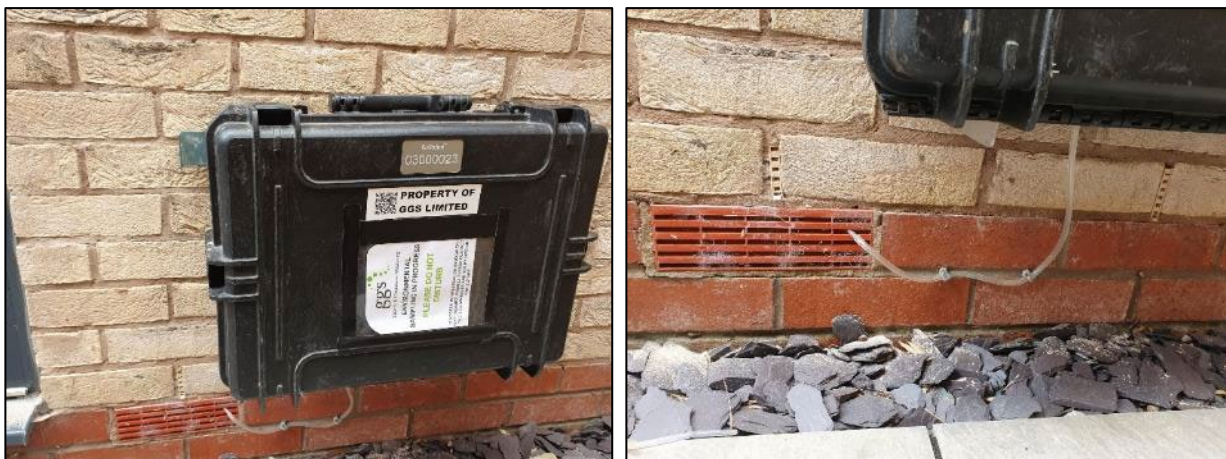
Figure 2 GGS site photographs of the Air Sentinel® instrumentation deployed at the Site. The instruments were secured to the walls and connected to the selected sub-floor void locations via air bricks using a length of semi rigid sample tubing.
