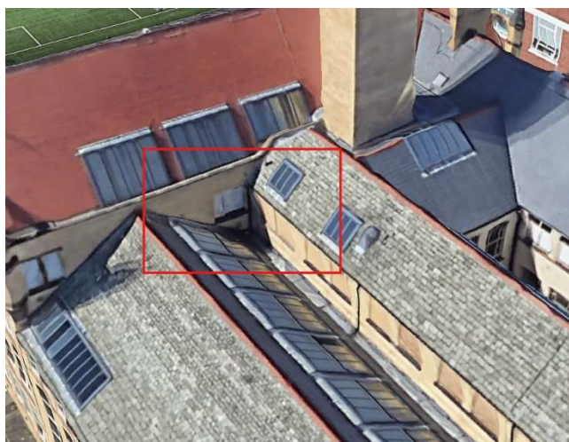
Location of new ladder – not visible from ground level*
