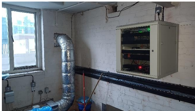
View within the roof mounted plantroom
