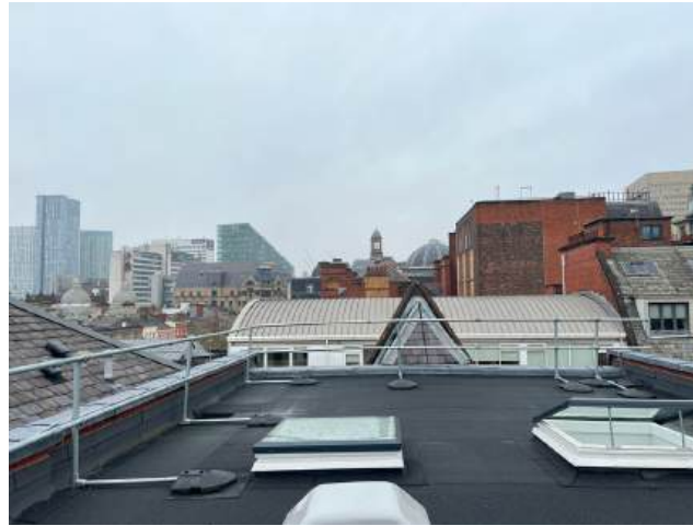
2.19 View towards King Street showing rooflights and services.heic
