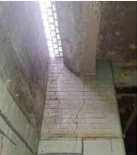
Figure 6 – Exemplary site photos of key conditions: concrete slab exposure, steel beam corrosion, cracking on surface
