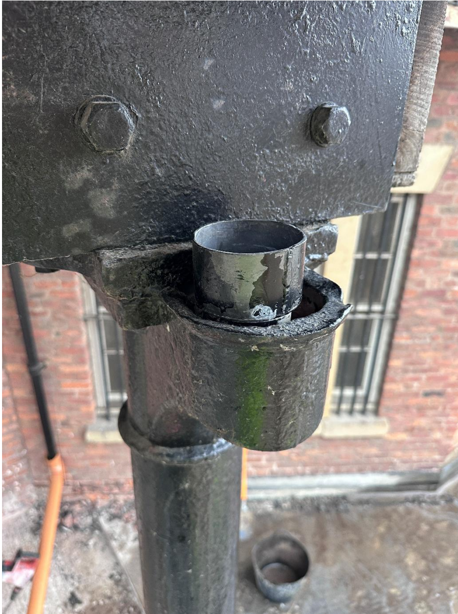
Photograph 3 – Head connection with internal column
