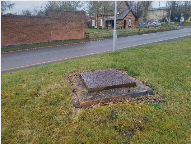
Figure 2.5: Raised man-hole covers in soft standing along the western boundary.
