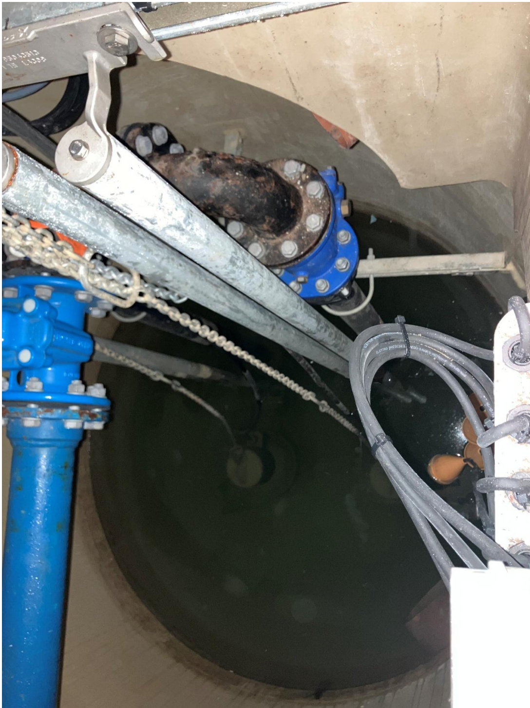
Figure 3 – Surface Water Pump Station Chamber - SPS1
