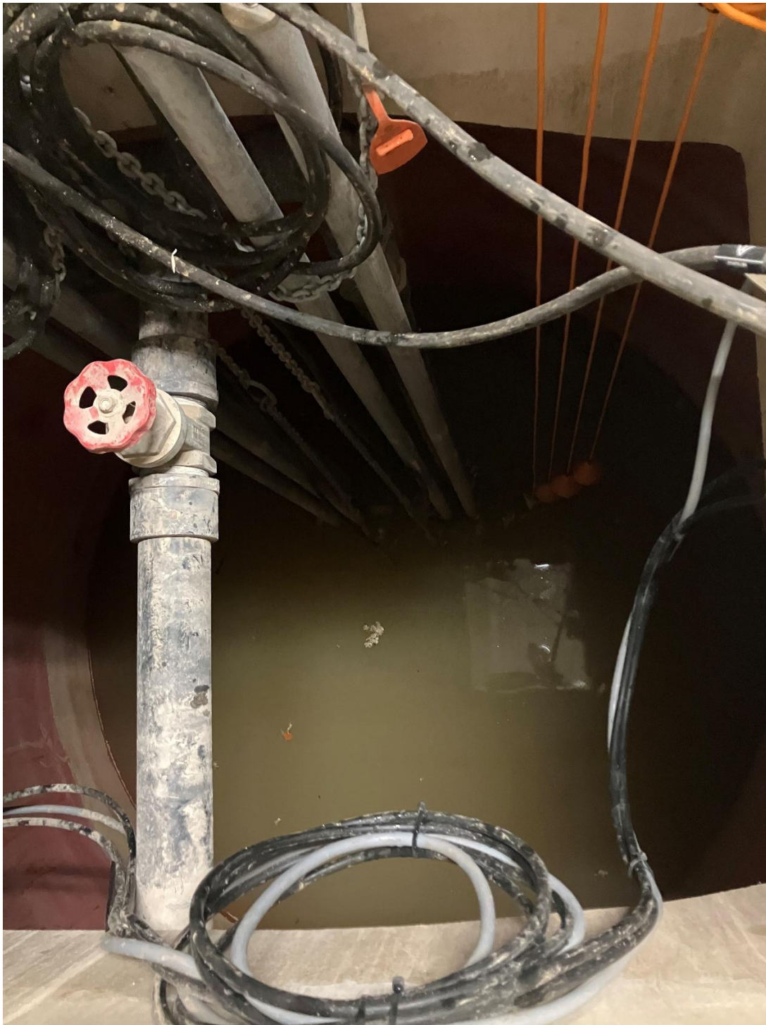
Figure 4 – Foul Water Pump Station Chamber – FPS1
