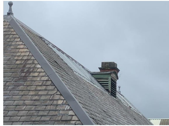
Picture 10 – Dilapidated dormer
