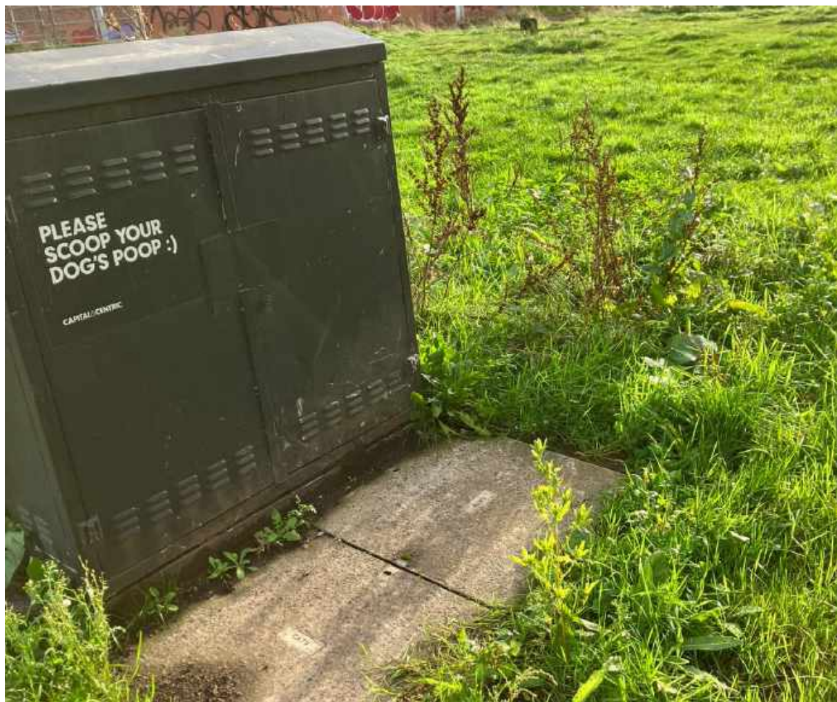
Photograph 5 – Broadband junction box located near the western boundary.
