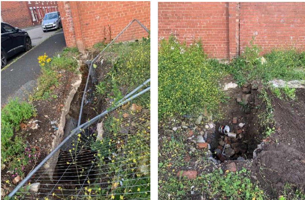
Figure 6: Photographs showing open holes along the southern boundary (left) and in the western site section (right).
