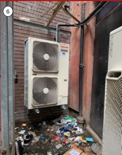
The current entrance is uninviting due to the M&E equipment next to the door and rubbish on the ground
