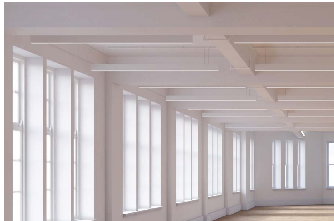
New linear lighting inbetween the cofferes
