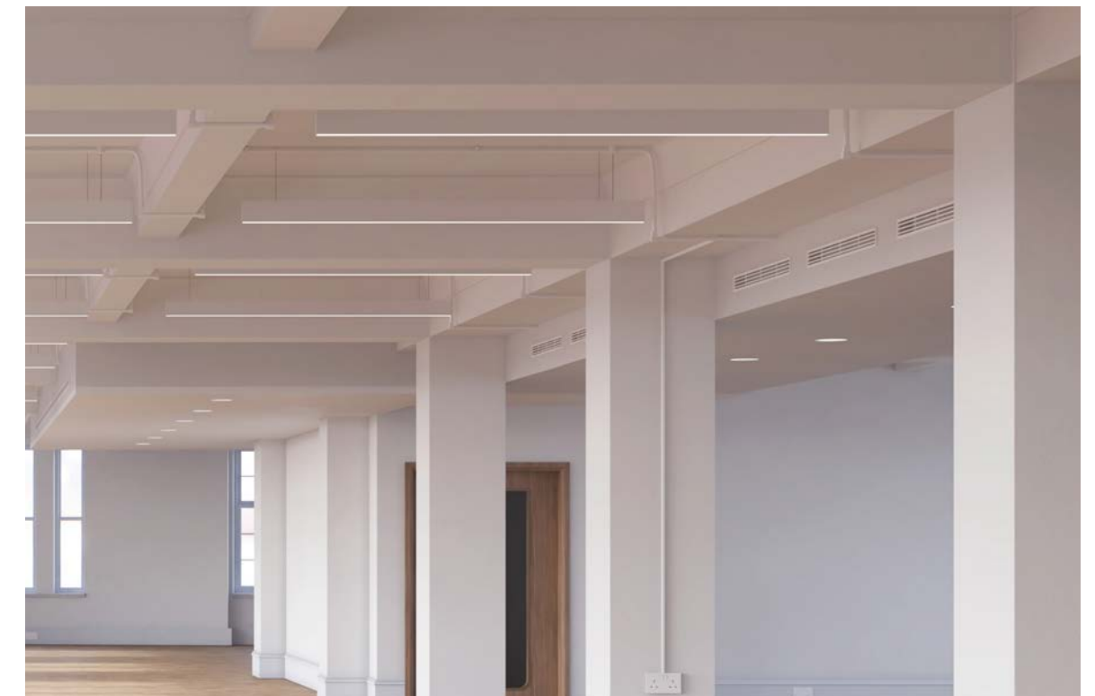
New central bulkhead with spotlights
