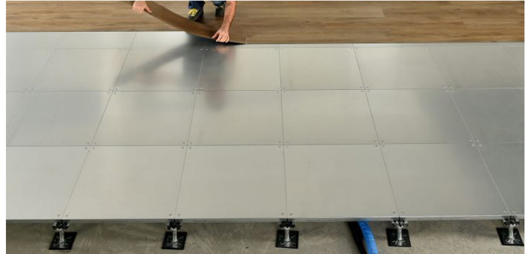
RAISED ACCESS FLOOR
