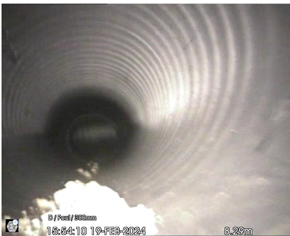
38X_7fd9689b-7494-4b8b-9ffd-75b43d27888f_20240220_131350_953.jpg, 00:00:36, 8.29 m Settled deposits, coarse, 5% cross-sectional area loss
