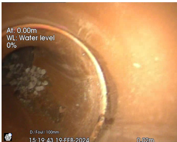
23X_c9193ec7-2856-419d-b543-537437b5a12a_20240220_130726_204.jpg, 00:00:16, 0.53 m Settled deposits, hard or compacted, 5% cross-sectional area loss, STONES UNABLE TO JET
