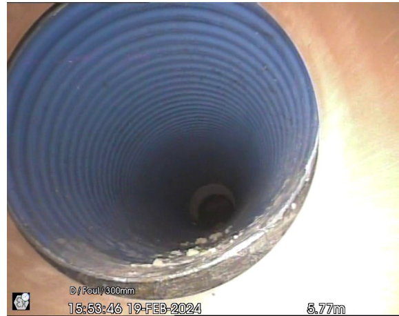
38X_a70927c2-bff9-48aa-8fd6-2b3f1407405a_20240220_131215_332.jpg, 00:00:26, 5.91 m Joint displaced, medium
