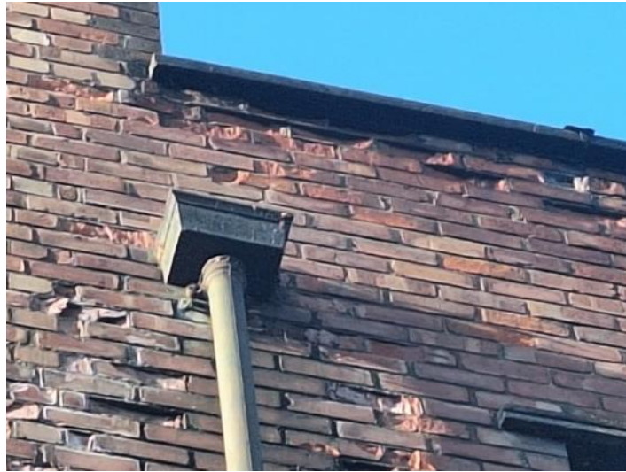
PLATE 2 SHOWING SUPERFICIAL DAMAGE AT TOP OF WALL PLATE
