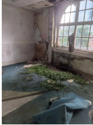
Photograph 8: Internal view of collapsed ceiling tiles on the top floor of the northern building at 4 Whitworth Street West.
