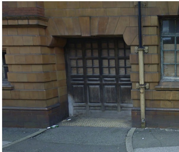
Photograph of the external substation door in original location
