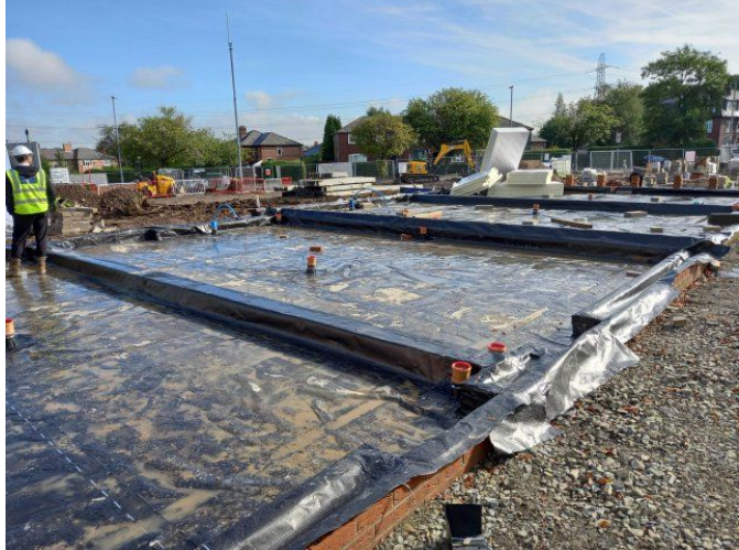
Evidence of gas membrane installed across Plots 1-4.
