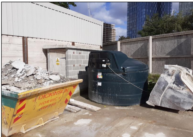
Figure 4.5 – Red Diesel tank (source: Heidelberg Materials)
