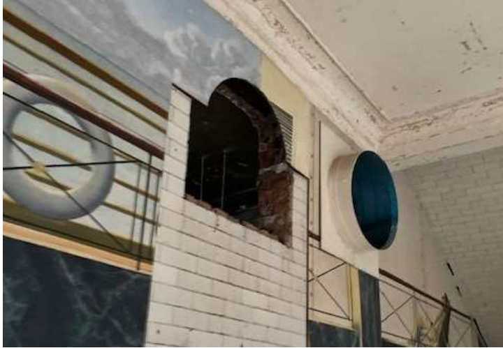
Figure 11 - Existing holes in tiled pool area
