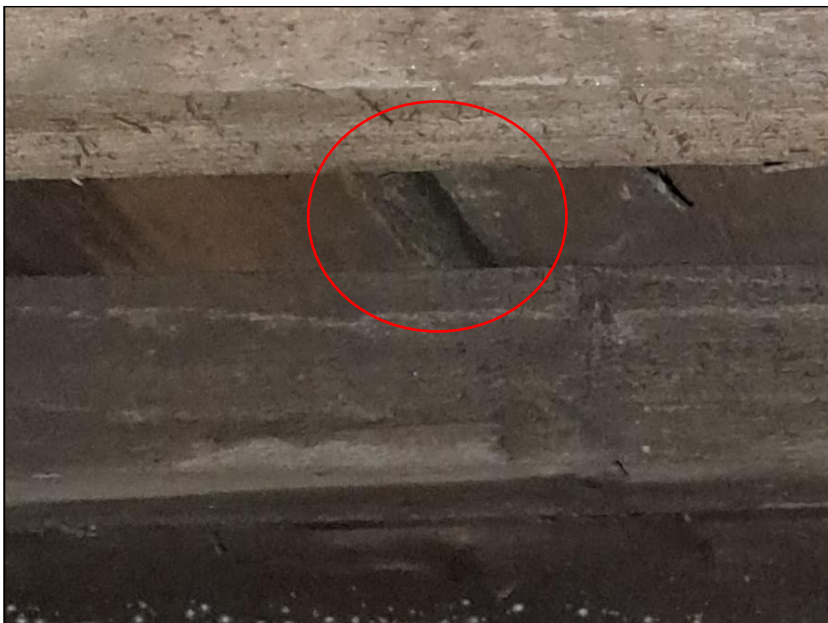
Photograph 12 showing a gap between the roof voids wooden sarking
