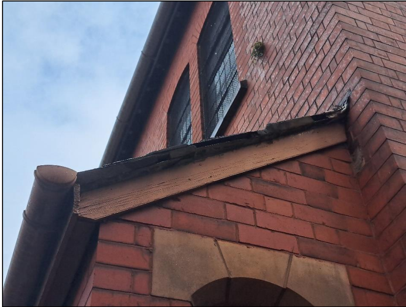
Photograph 3 showing the gaps in the mortar line
