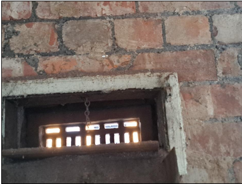
Photograph 9 showing one of the ventilation grilles
