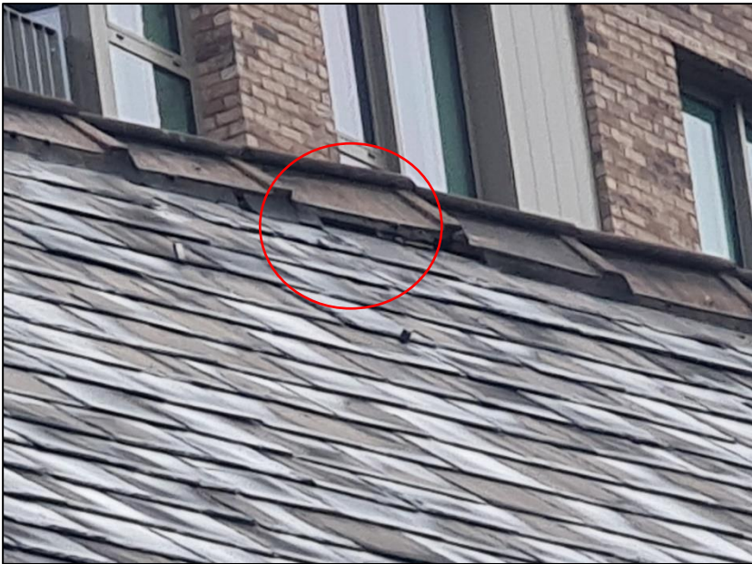
Photograph 6 showing a gap under a ridge tile
