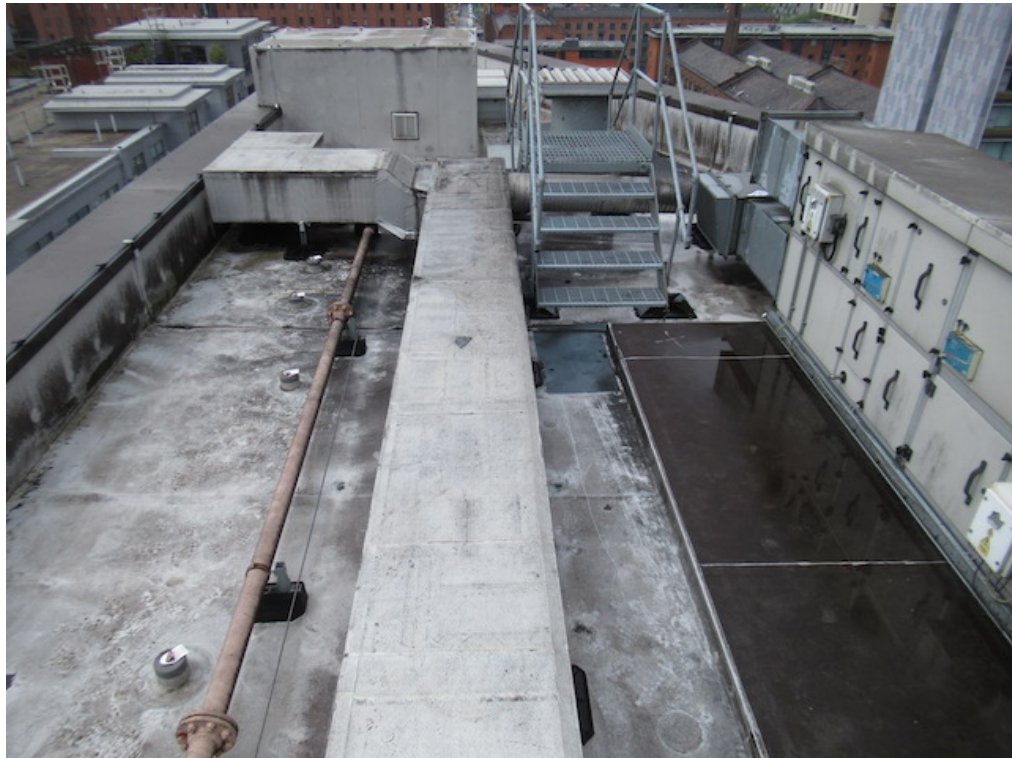
5. General view of AHUs and ductwork to main roof
