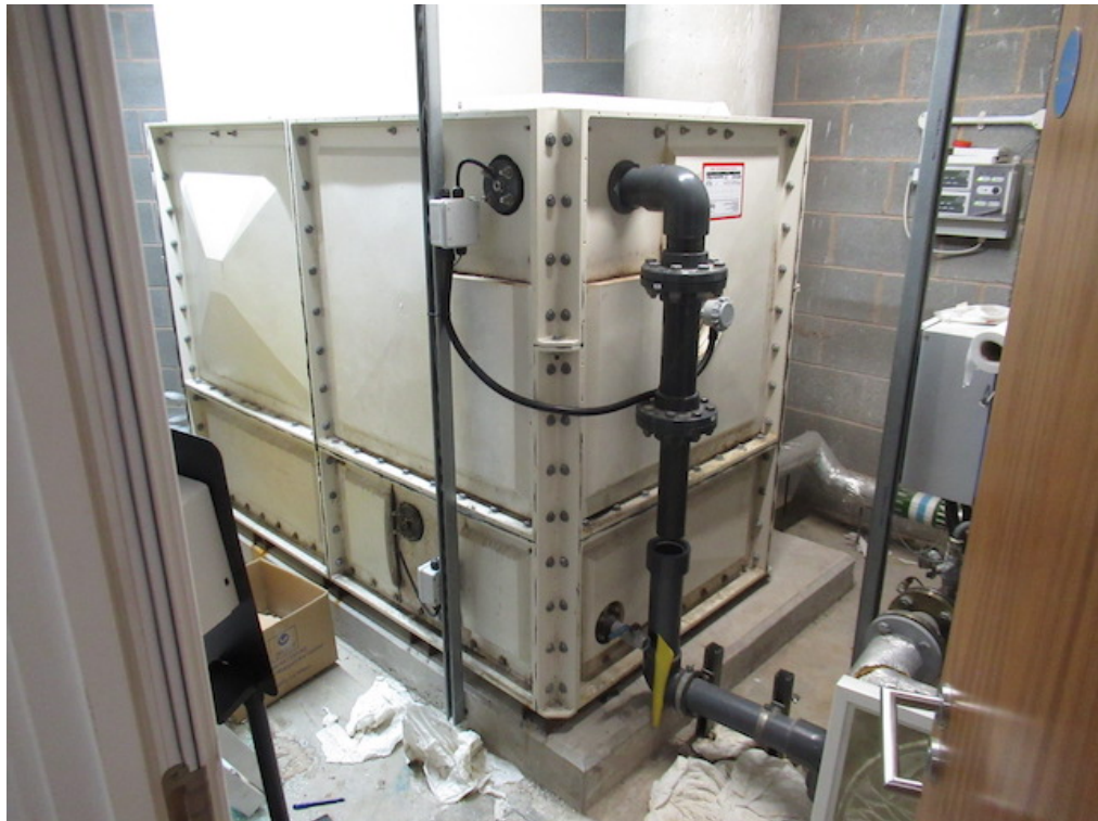
18. General view of water/pumps room equipment to basement
