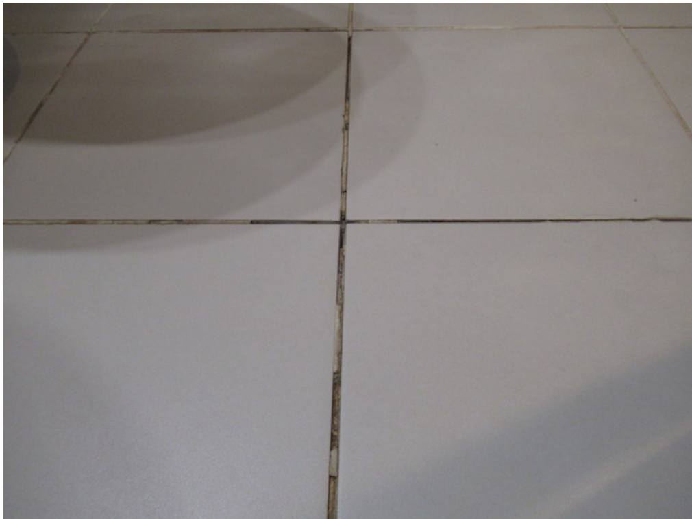
24. Poor condition of floor grout to bathroom pods
