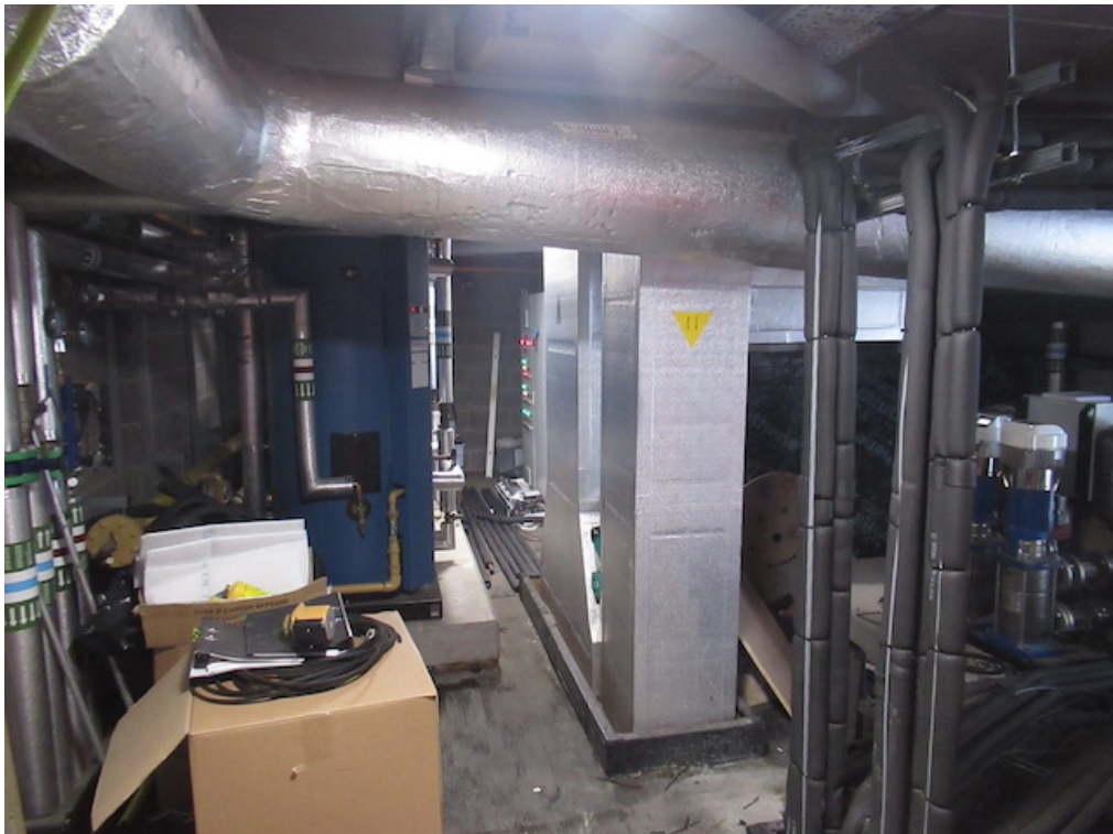
8. General view of equipment to roof level plantroom
