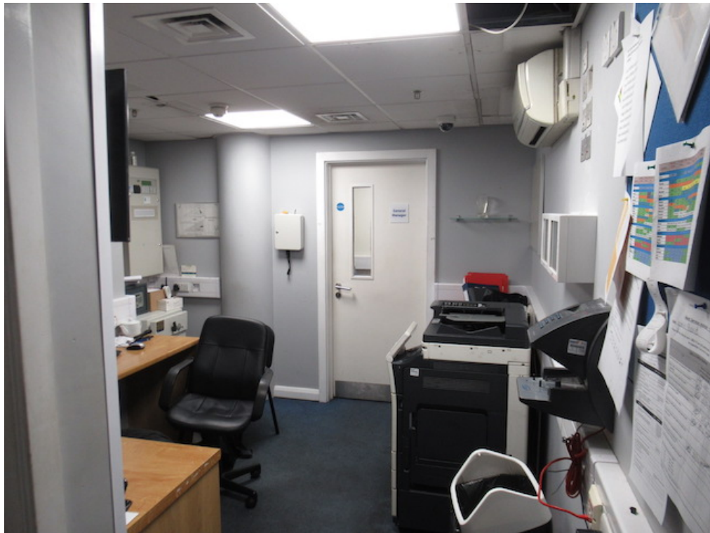
14. Typical worn finishes to 'back of house' offices
