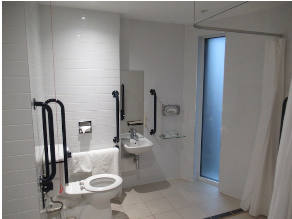
25. Fair condition of finishes to 'accessible' bathrooms
