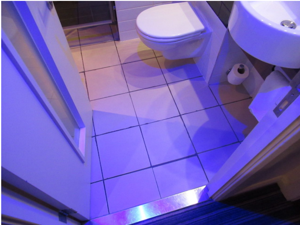
23. Poor condition of floor tiles and grout to bathroom pods
