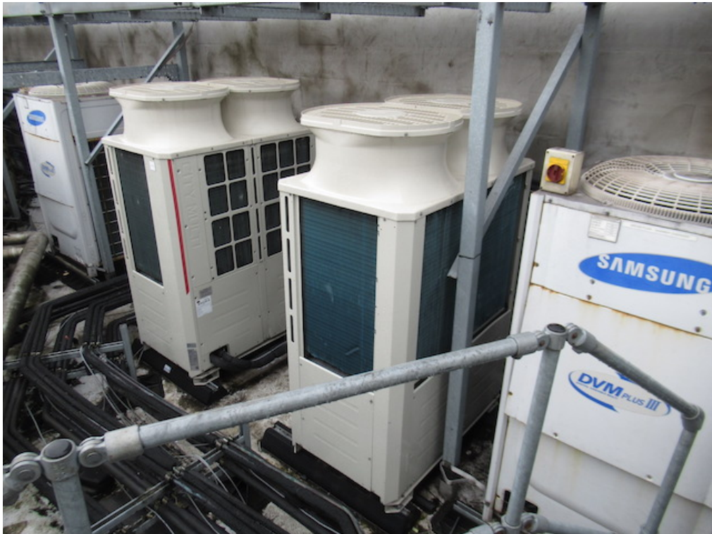
7. General view of original and replacement condensers to main roof
