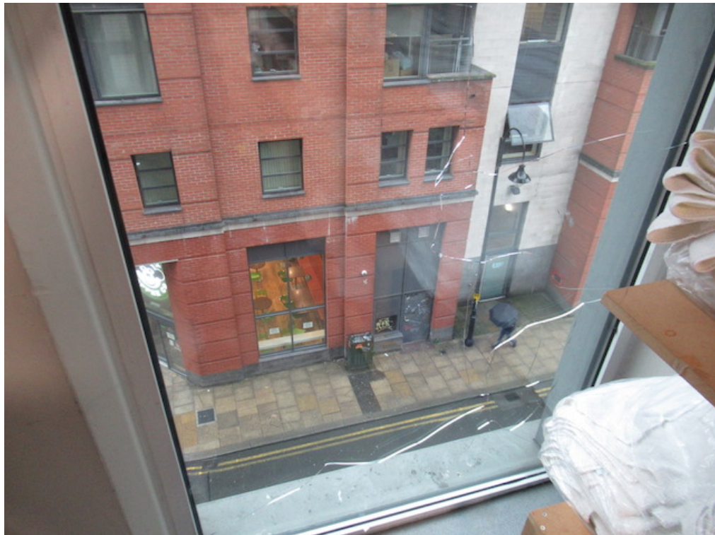
26. Typical smashed inner panes to linen store windows
