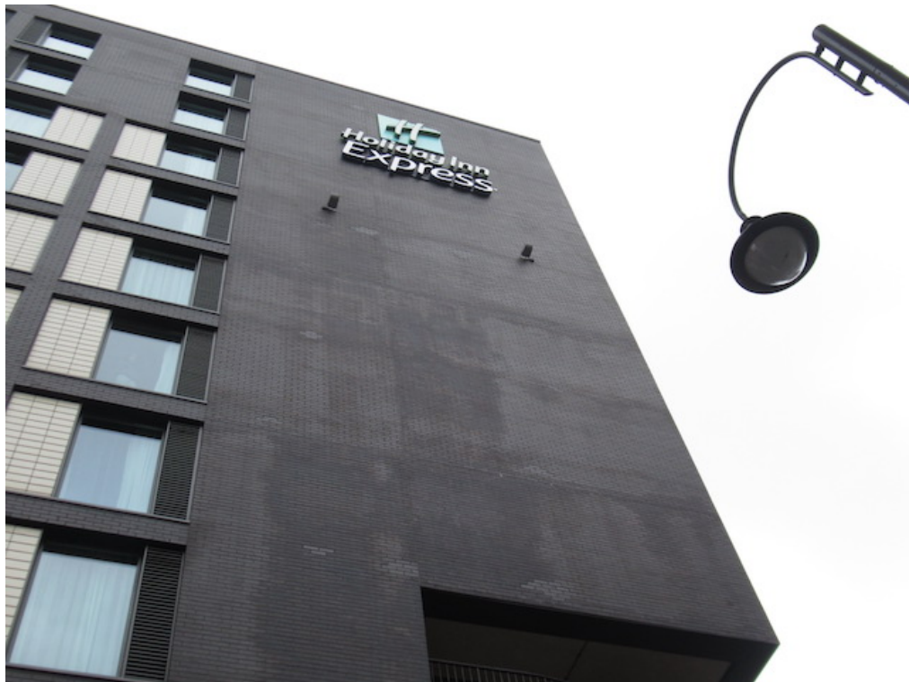
9. Mismatched brickwork to right side of Hulme Street elevation
