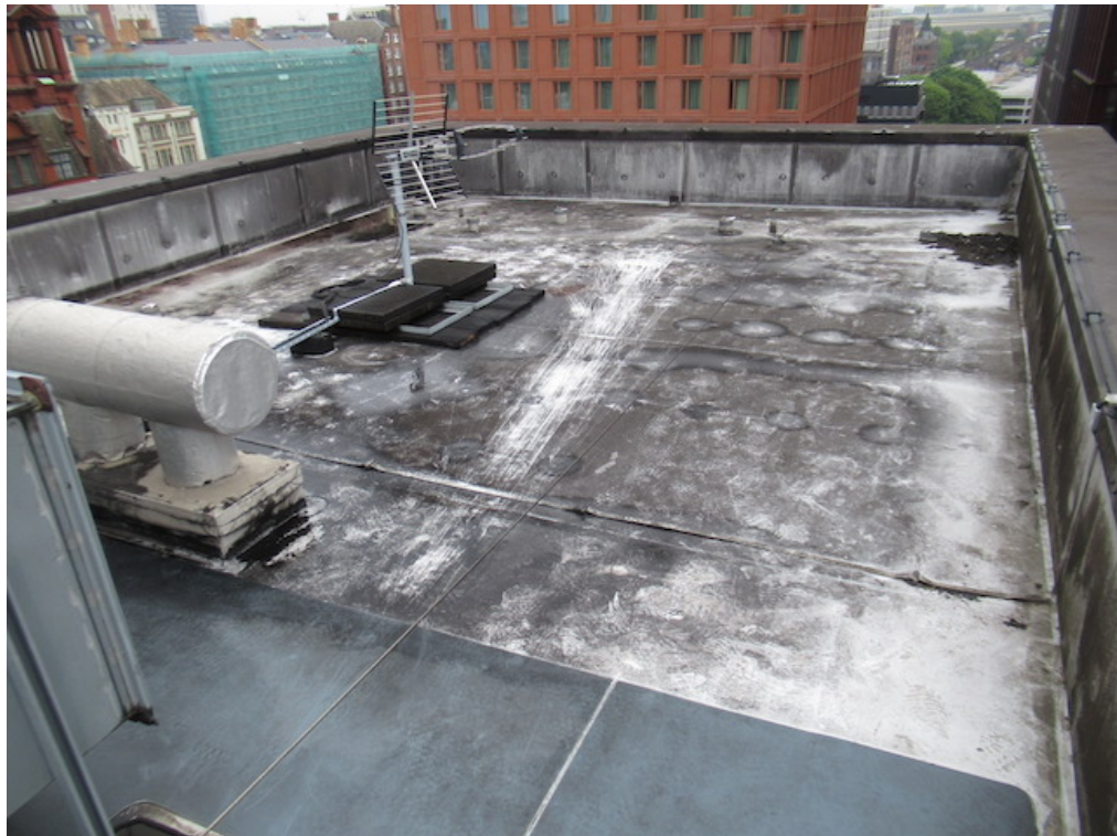
4. Typical soiling throughout flat roofs
