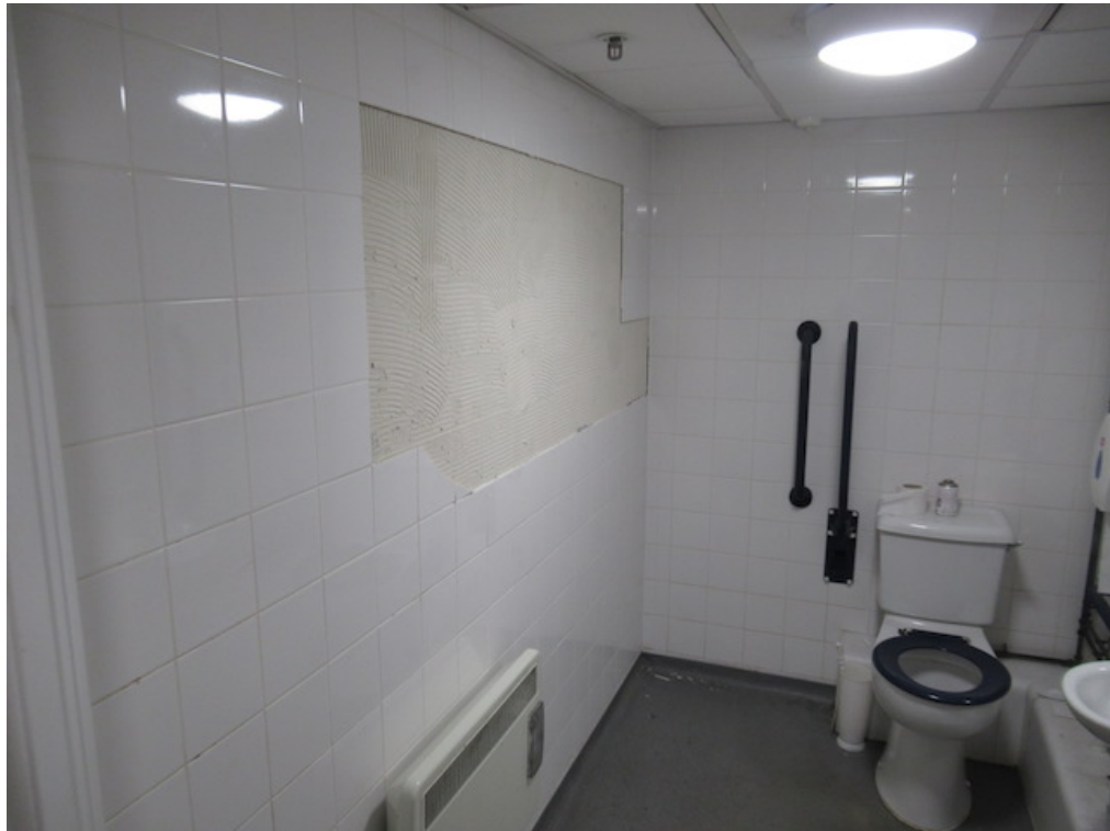
17. Absent and debonded tiles to male staff changing areas / toilets
