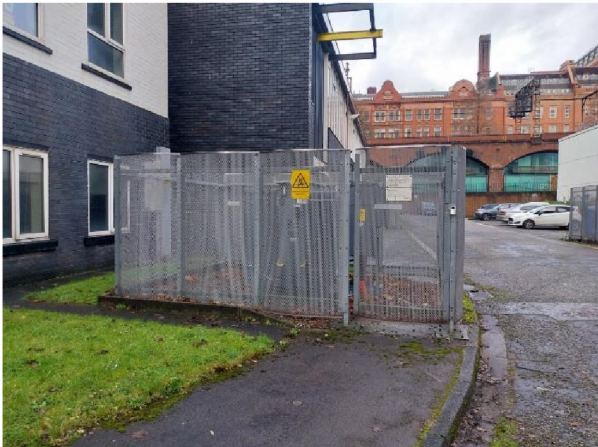
25. Electrical substation to rear of Paper Science, facing north
