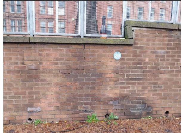
32. Cracking of Vimto Gardens retaining wall, facing north
