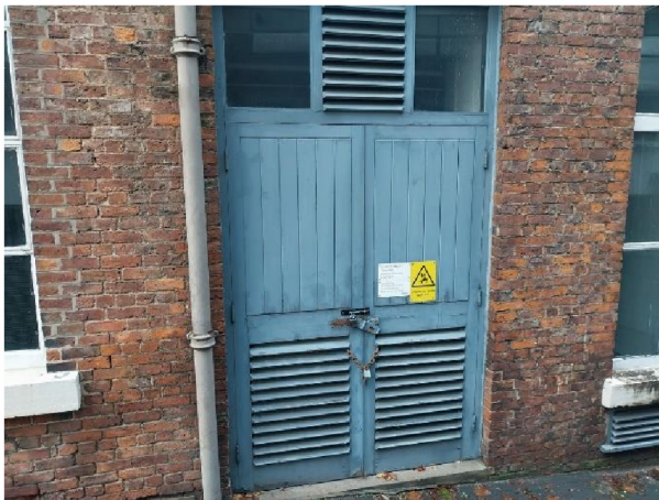
9. The Mill electrical substation
