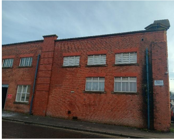
Figure 8: Photograph of staining from rainwater discharging against the facades as a result of deficient/unmaintained rainwater goods. Source: SLHA 2024
