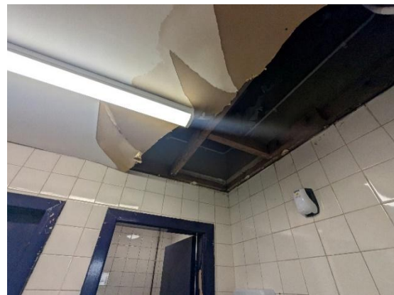
Figure 11: The ceiling finishes of the Driver's Area female toilets have come away due to water penetration issues at roof level/ Source: SLHA 2024
