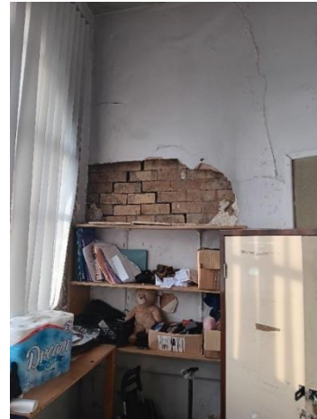
Figure 9: View of the structural crack within the Lost & Found Office in the front administrative range. Source: SLHA 2024
