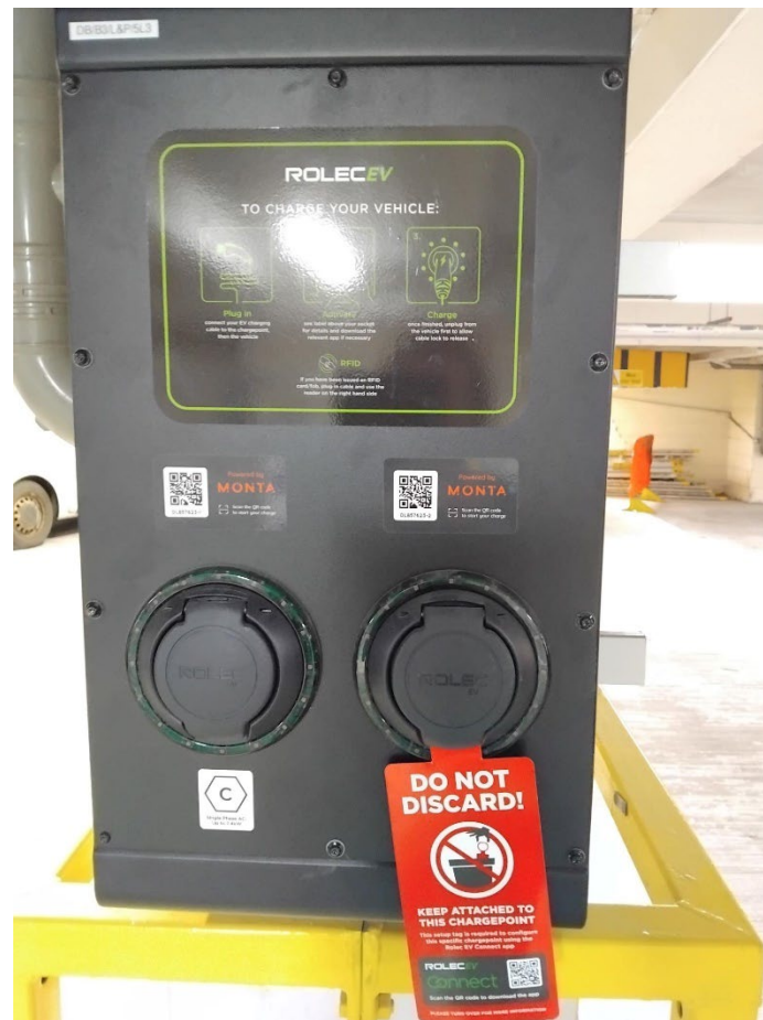
Figure 1. Photographic Evidence – EV Charger
