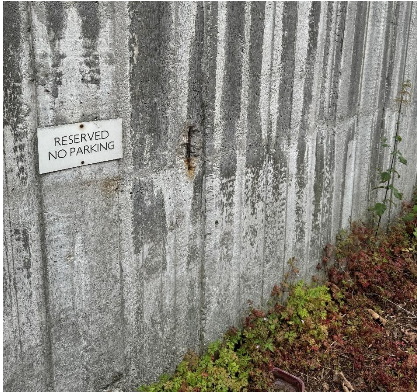
Figure 19: Signage fixed to the inside face of the Wall along with exposed reinforcement (2024)
