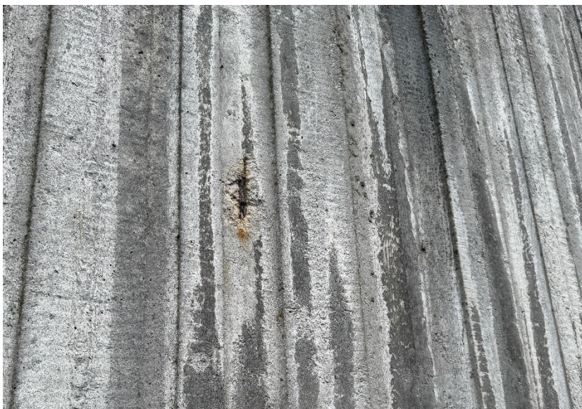
Figure 18: Further signs of exposed reinforcement (2024)
