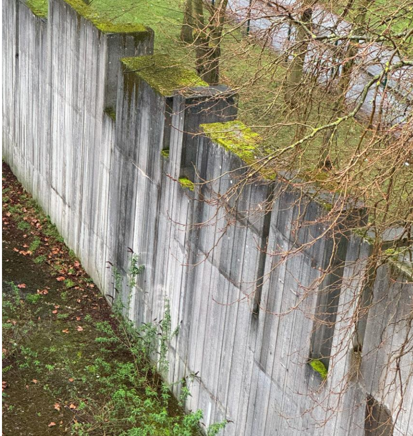
Figure 25: Moss and vegetation evident atop the Wall (2024)
