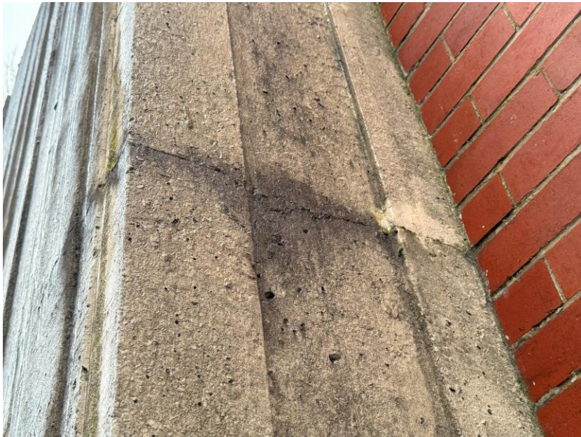
Figure 20: Cracking evident at northern Wall edge (2024)
