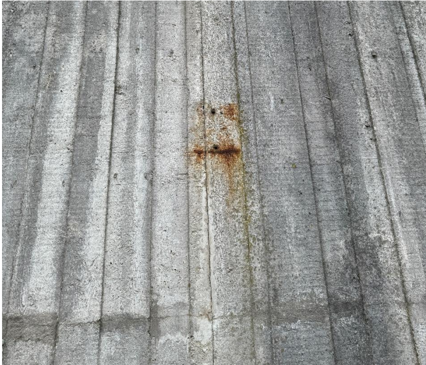
Figure 23: Rust stains thought to be from previous steel canopy structure (2024)
