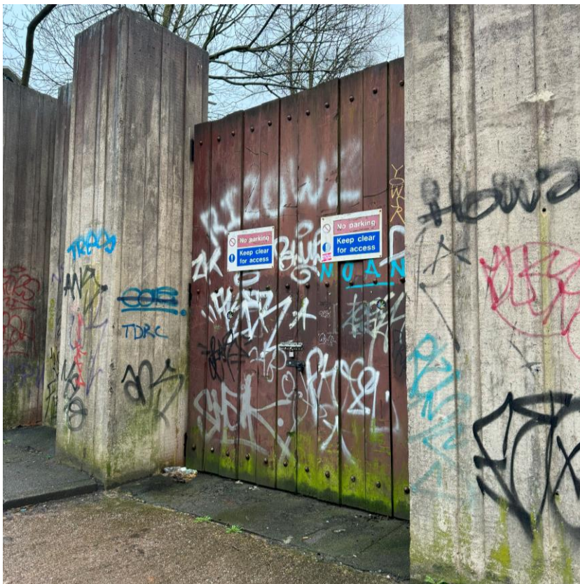
Figure 24: Graffiti to the accessible Altrincham Street facing elevation (2024)
