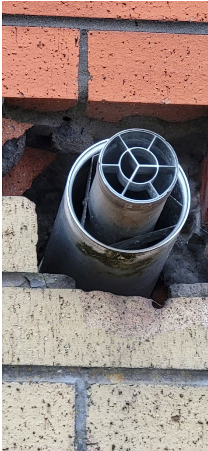
FIGURE 11 GAP AROUND HEATING VENT - ACCESS POINT FOR BATS INTO THE VOID BEHIND THE BRICKWORK
