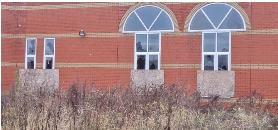
FIGURE 10 BROKEN WINDOWS – ACCESS POINT FOR BATS INTO THE MAIN BUILDING
