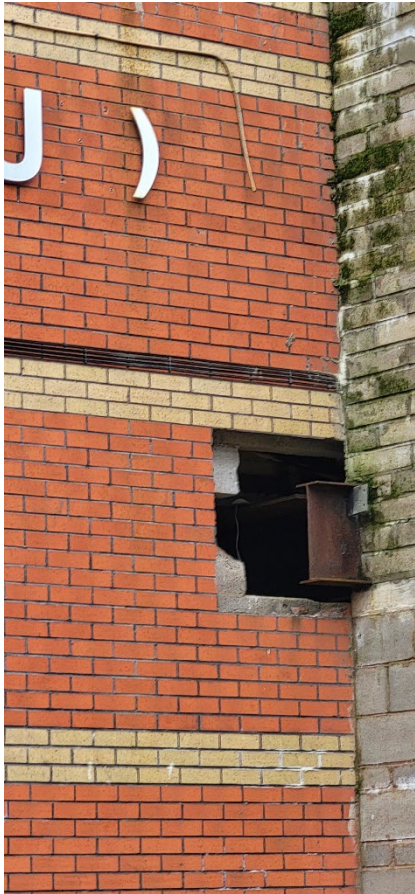
FIGURE 9 HOLE IN BRICKWORK - ACCESS POINT FOR BATS INTO THE MAIN BUILDING
