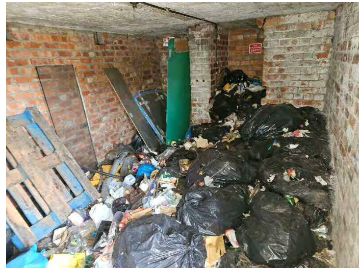
Photograph 8 – A view of the waste materials within the outbuilding in the eastern corner of the site.
