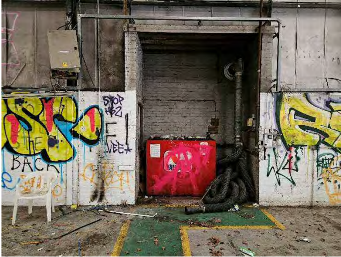
Photograph 13 – A view of the above ground fuel/waste oil tank within the internal vehicle maintenance area.
