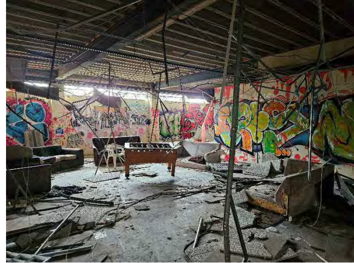
Photograph 14 – A view inside the vandalised and derelict welfare and administration area in the western part of the building.
