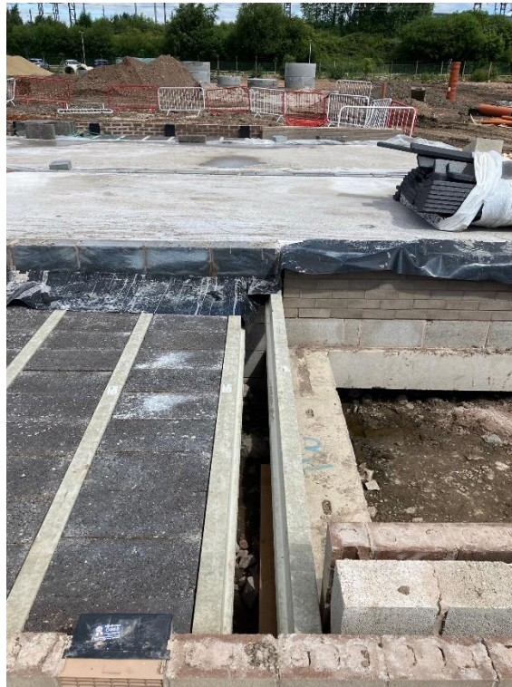
Plate 3 – Membrane present below floor screed – to be extended below garage
