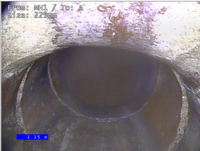
Line of drain/sewer deviates up - Remark: SHARP
