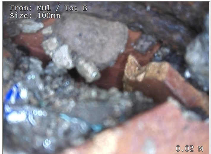
Survey abandoned - Remark: DUE TO COLLPASE
