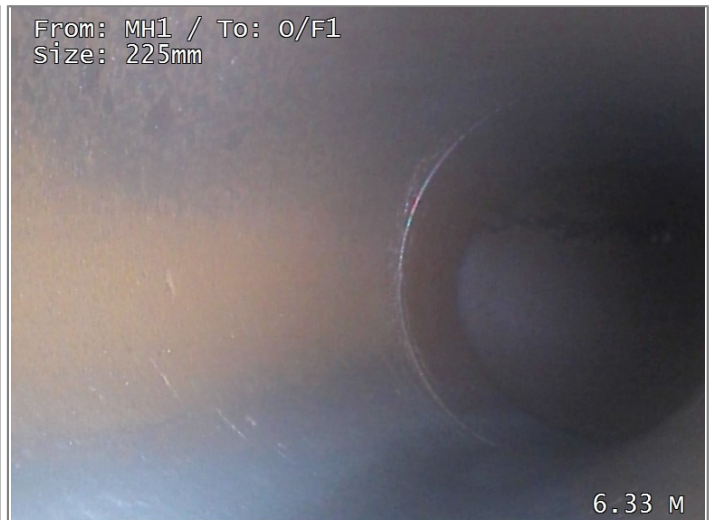
Line of drain/sewer deviates right
