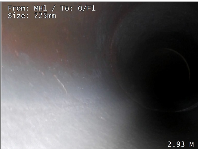
Line of drain/sewer deviates right
