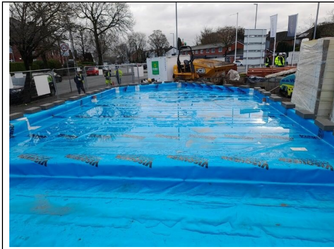
Evidence of Visqueen gas membrane installed across the southern part of the apartment building.
