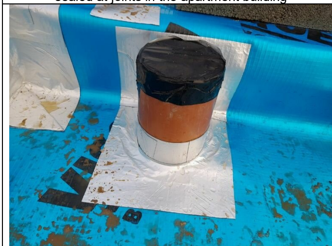
Evidence of sealing at service entry points in the apartment building
