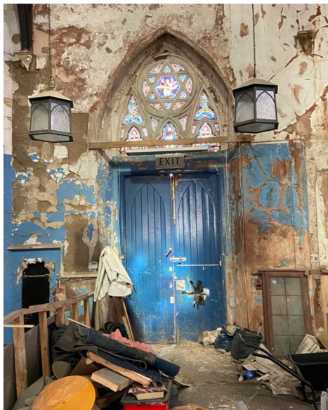
Damaged plaster to perimeter walls
