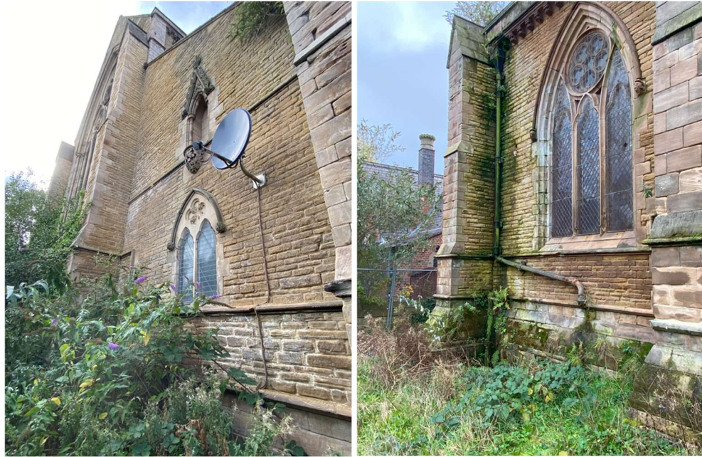
South facing elevation and damaged rainwater pipes
