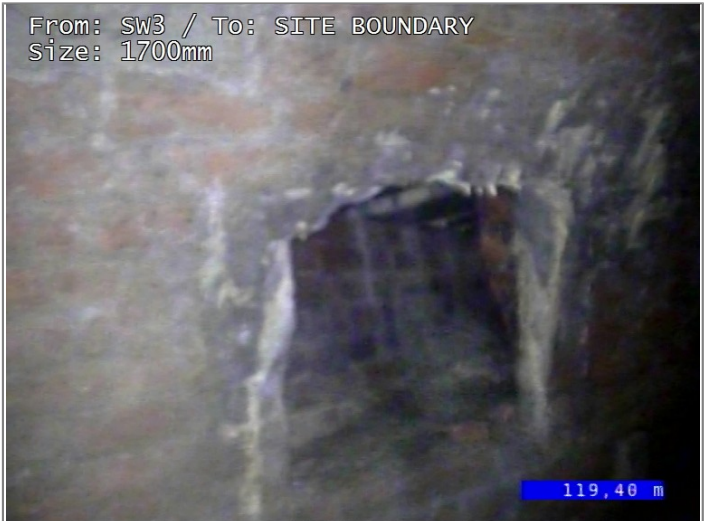
Junction at 9 o'clock, diameter 450mm
