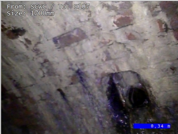
Junction at 4 o'clock, diameter 150mm
