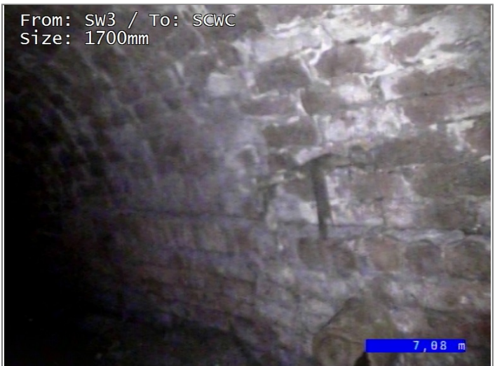
Connection other than junction at 5 o'clock, diameter 150mm
