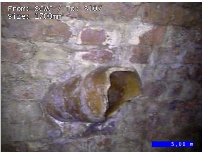
Connection intruding at 9 o'clock, diameter 150mm, intrusion 5%
