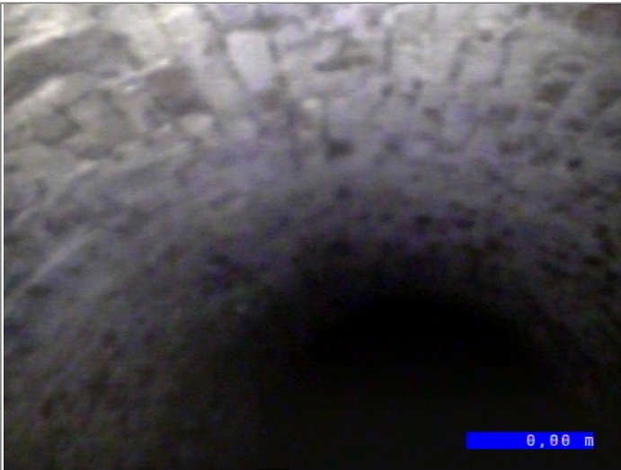
Start node type, manhole, reference SW3
