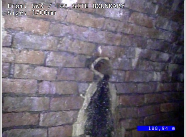
Connection other than junction at 8 o'clock, diameter 150mm
