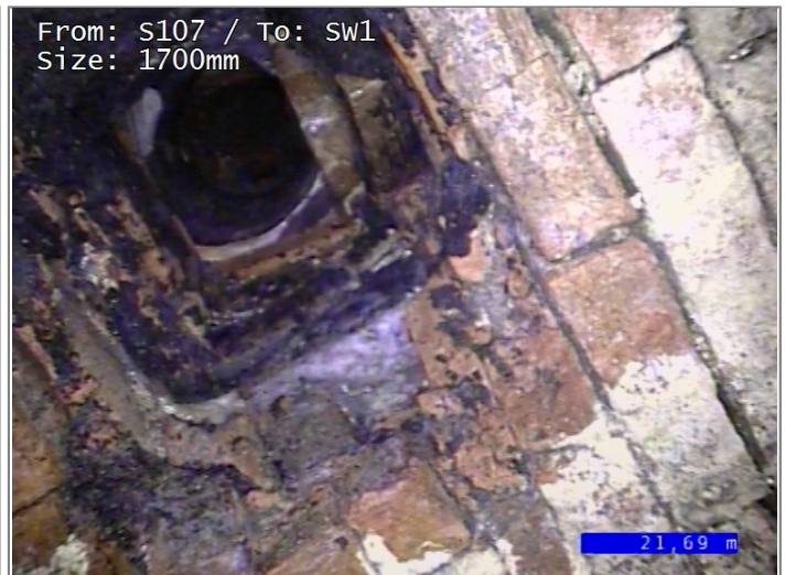
Junction at 12 o'clock, diameter 225mm
