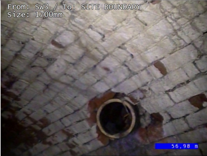
Connection other than junction at 3 o'clock, diameter 225mm
