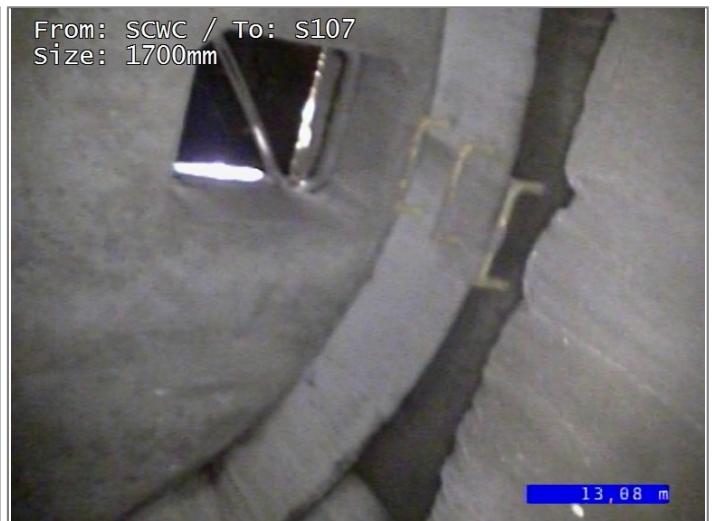
Finish node type, manhole, reference S107
