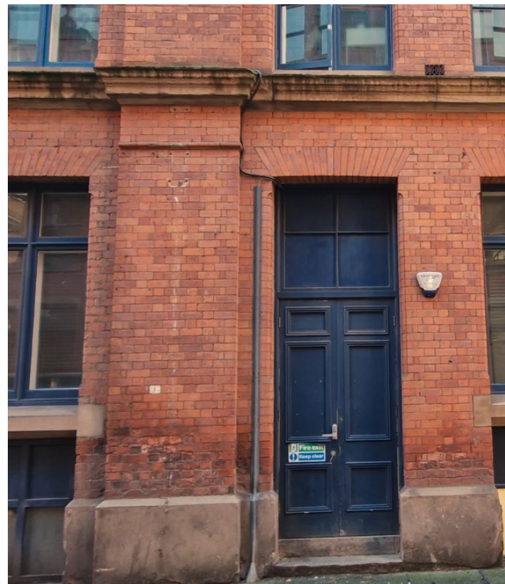
Plate 23: Evidence of former fittings in the location of the proposed projecting sign.
