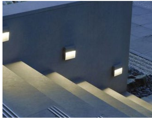
Wall mounted lighting to cast light wash across steps
