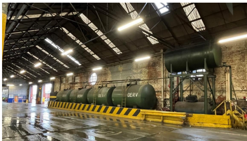
Figure 7: Existing fuel/coolant tanks
